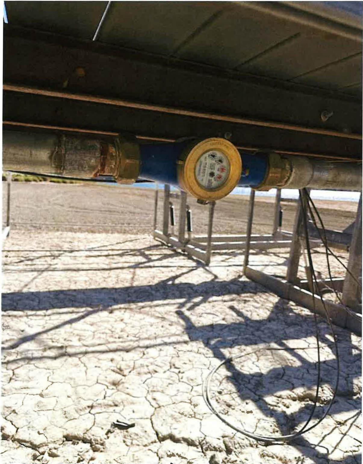
FLOWMETER INSTALLED AS PART OF DIVERTING WORKS
