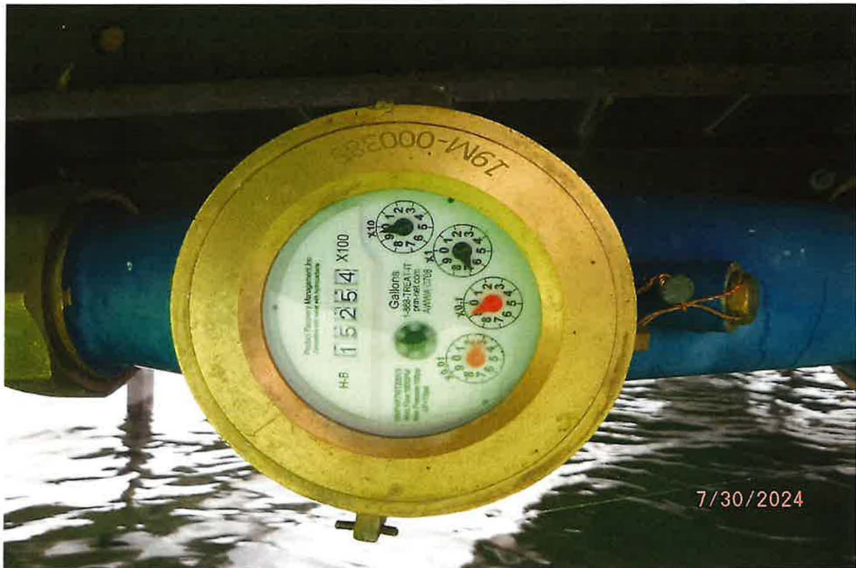
PRM - FLOWMETER INSTALLED IN-LINE BENEATH DOCK PRIOR TO SYSTEM'S PRESSURE POT
