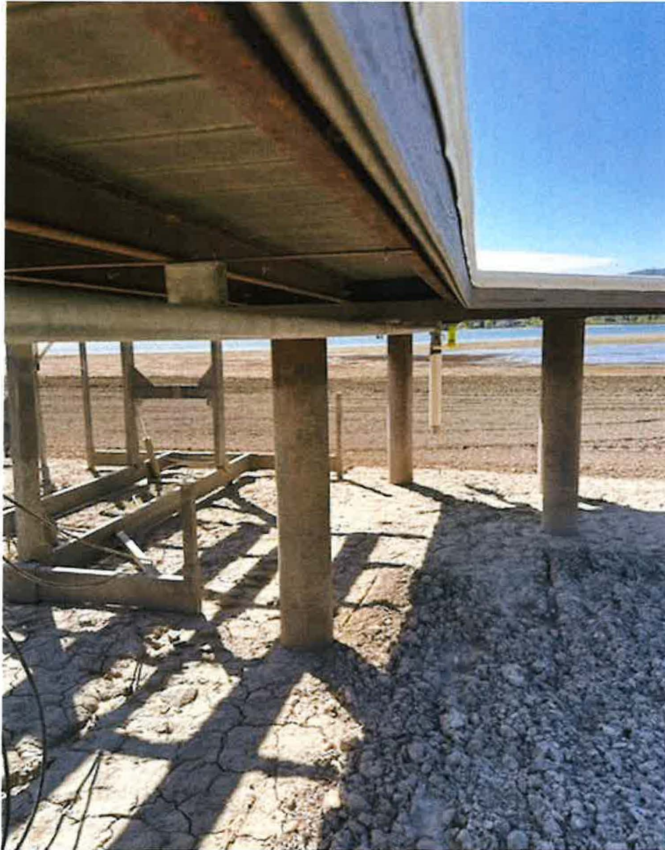
2-INCH PIPELINE ROUTES BENEATH DOCK UNTIL SHORELINE WHERE IT IS BURIED TO IRRIGATION SYSTEM
