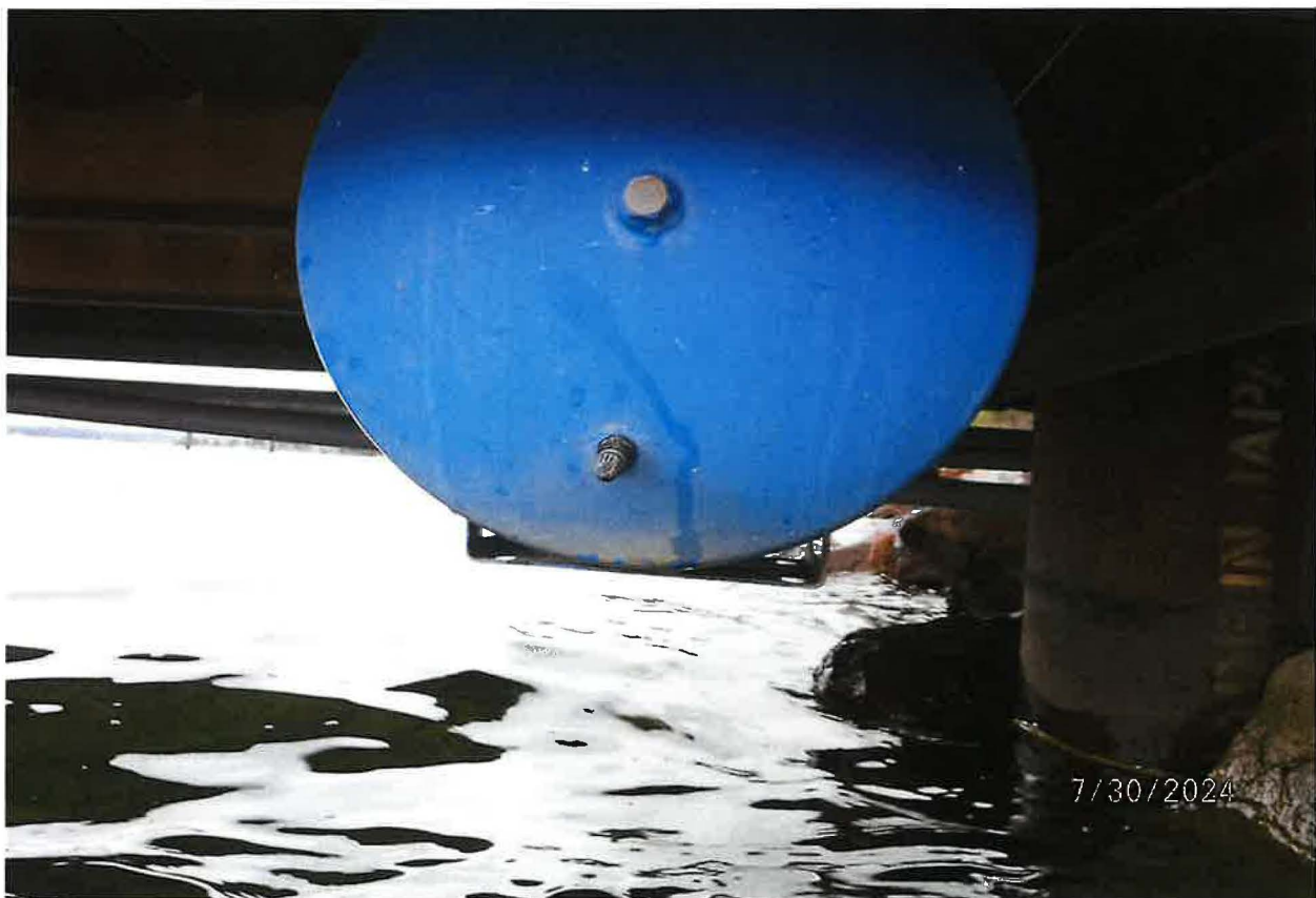
PRESSURE POT INSTALLED ON DIVERTING WORKS – LOCATED BENEATH DOCK AT SHORELINE
