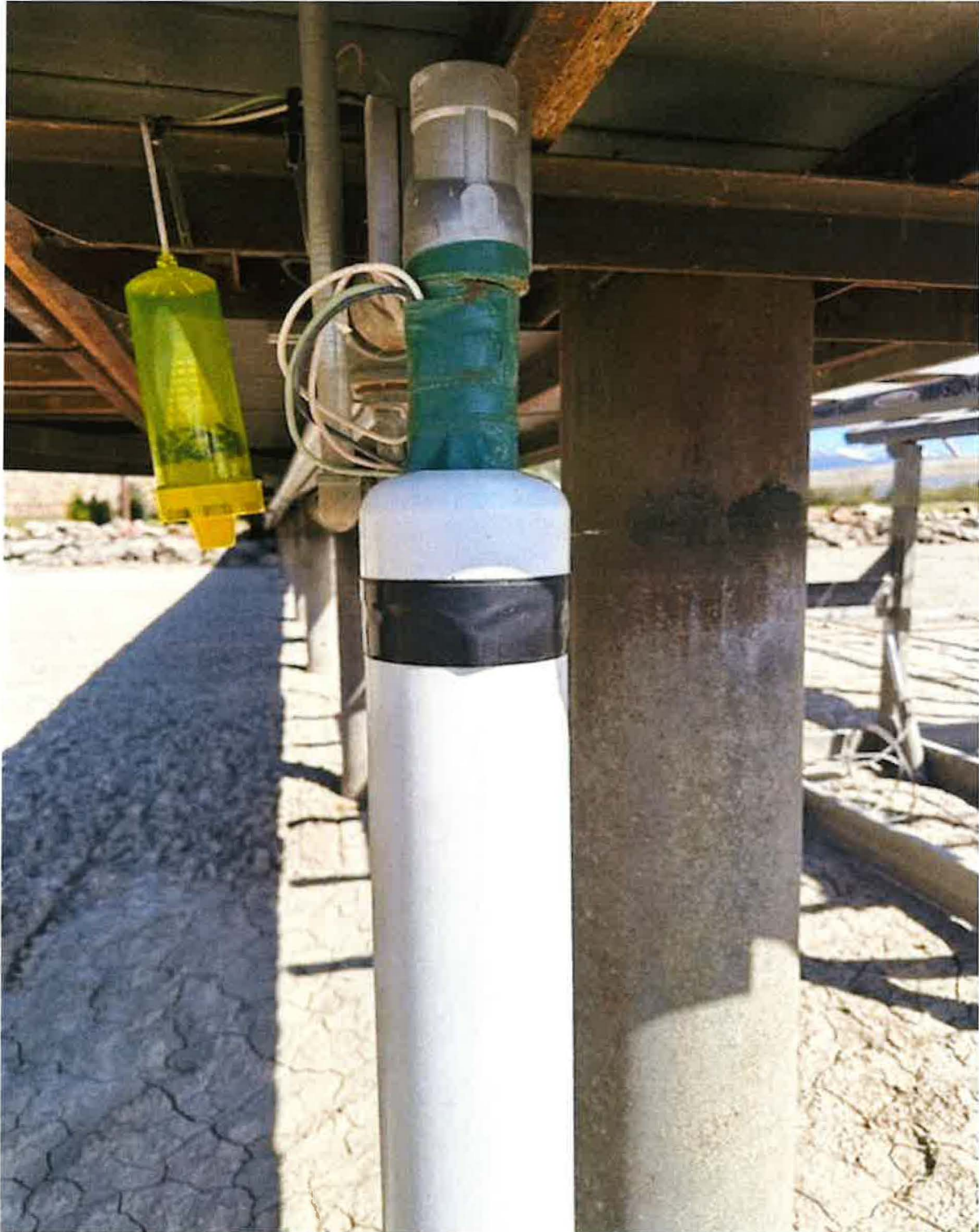
SUBMERSIBLE PUMP ENCLOSED IN PVC PIPE WITH SCREEN
