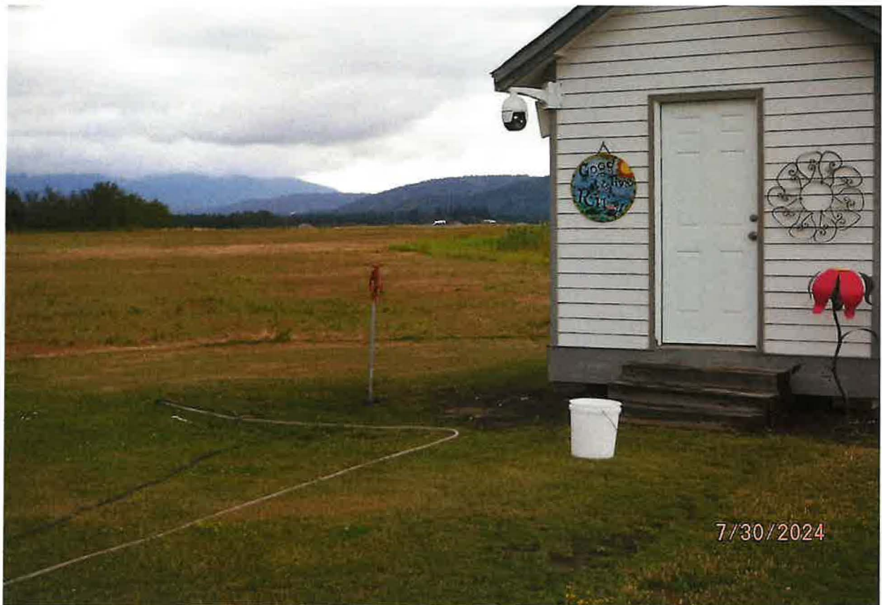
PUMP STATION & RED HANDLED FROST-FREE HYDRANT LOCATED BEACHFRONT IN THE IRRIGATION POU
