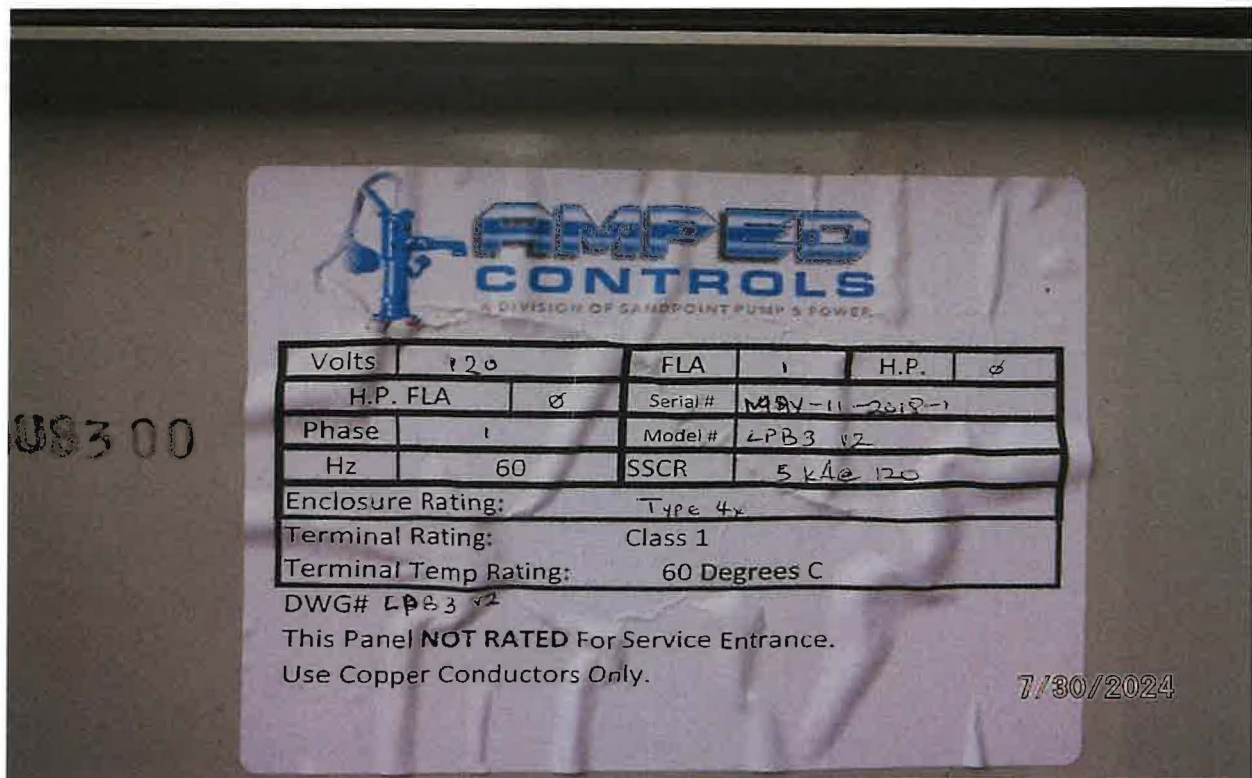
AMPED CONTROLS – CONTRACTOR WHO INSTALLED THE WATER SYSTEM; 1 HP PUMP
