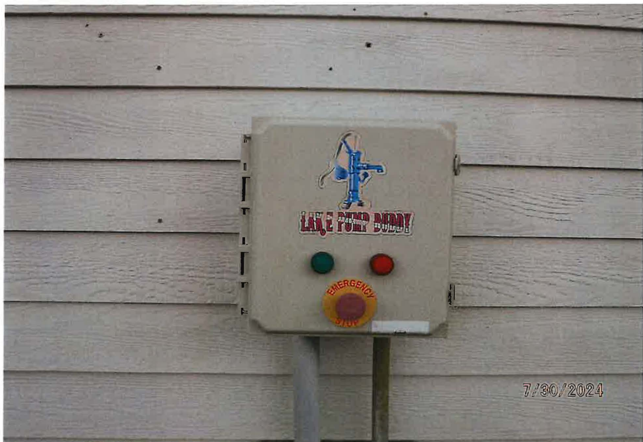
EMERGENCY SHUTOFF PANEL
