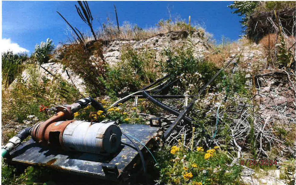
CONVEYANCE SYSTEM – 2-INCH FLEXIBLE PIPELINE ROUTED UPGRADE 30-FT ELEVATION GAIN PRIOR TO DISTRIBUTION TO IRRIGATION & STOCKWATER SYSTEMS
