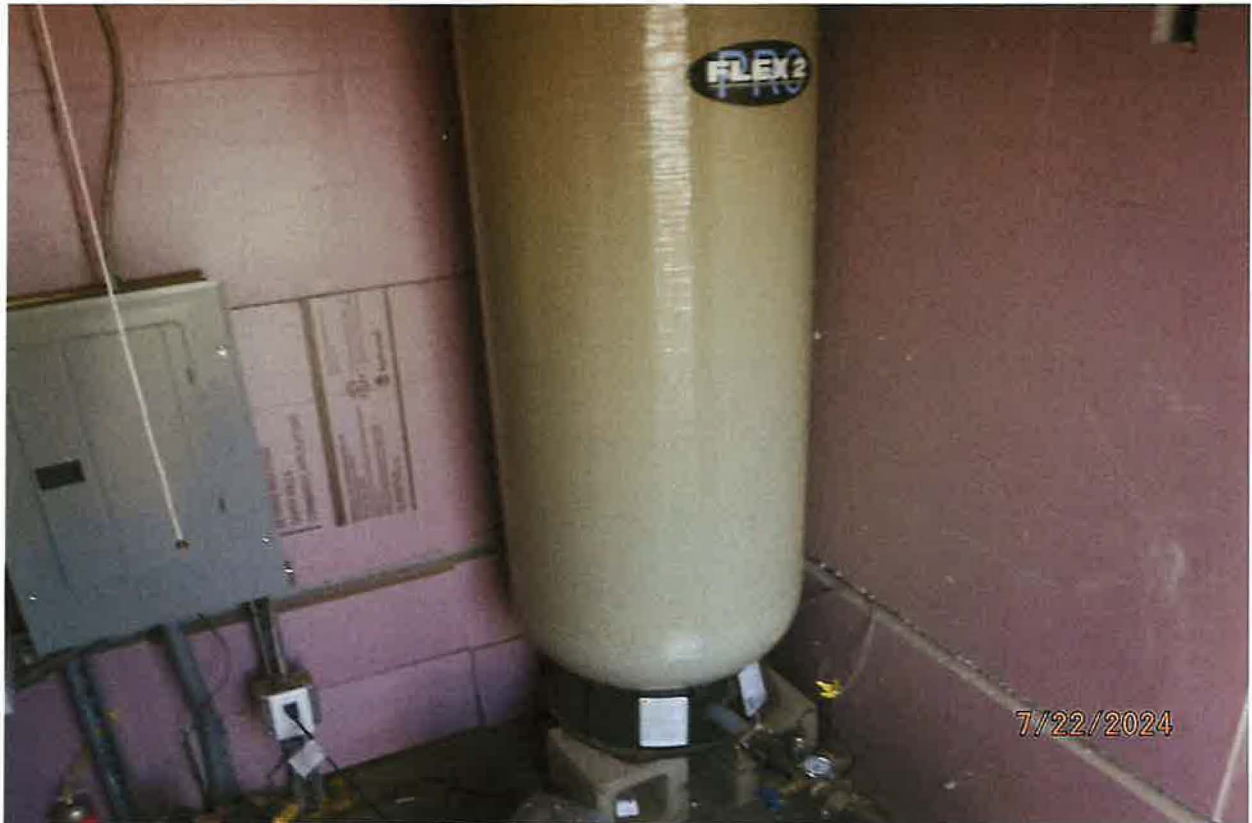
WELL PUMP ROUTES DIRECTLY TO PRESSURE TANK BEFORE DISTRIBUTION TO IRRIGATION SYSTEM
