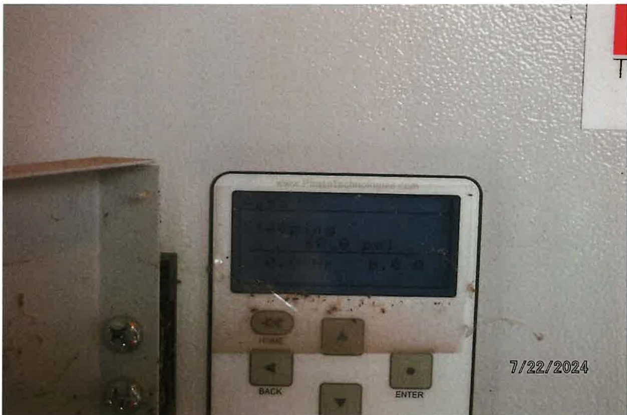
WELL PUMP CONTROLLER – PHASE TECHNOLOGIES MODEL 2XD210R-OFS. CONVERTS SINGLE PHASE TO THREE PHASE POWER
