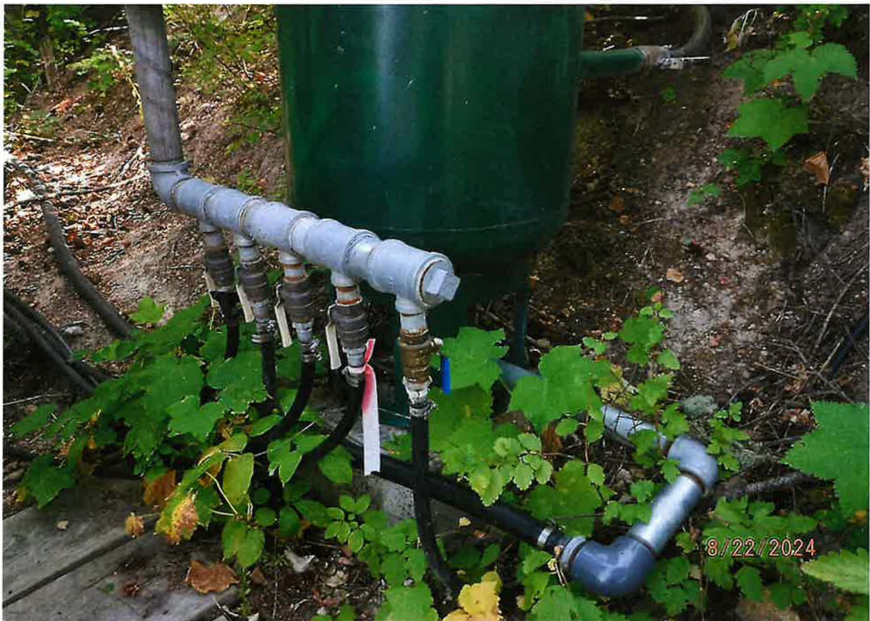
METAL FILTRATION SYSTEM AND DISTRIBUTION WATER LINE MANIFOLD – GRAVITY FLOW SYSTEM
