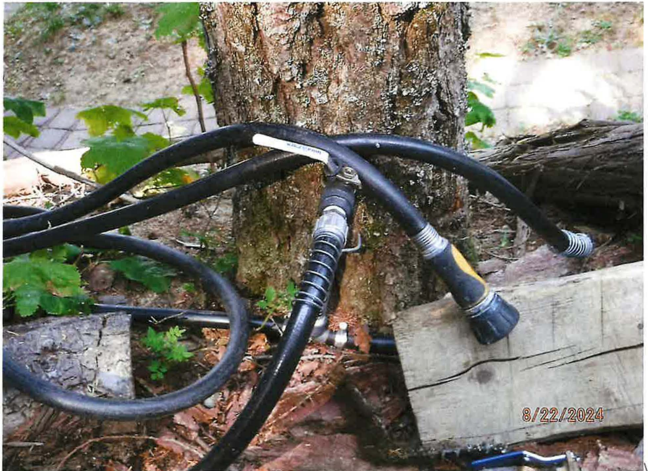
IRRIGATION POU – LOT 22, BLK 1; MULTIPLE HOSE TO SPRINKLER ATTACHMENTS FOR LANDSCAPE WATERING AND TREE WATERING
