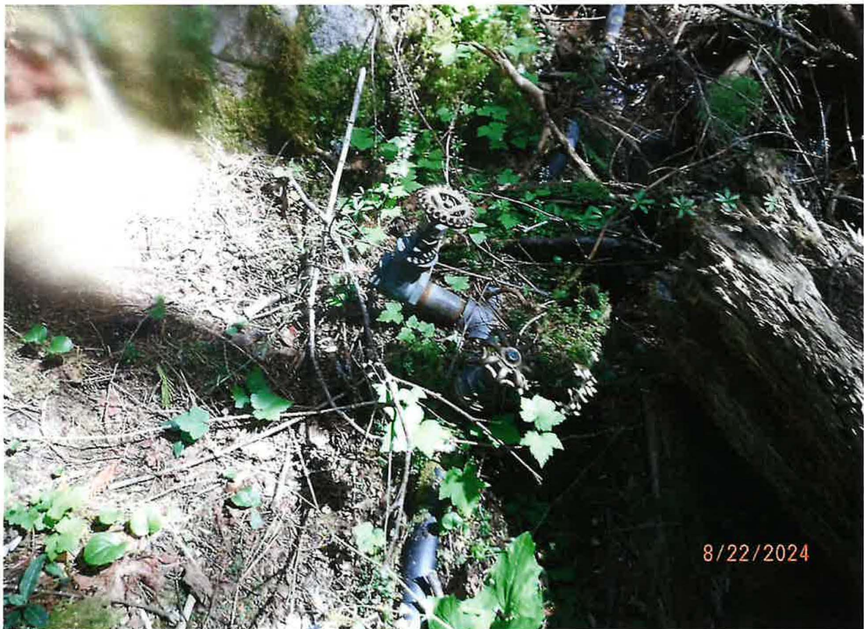
ONE OF THREE PRIMER/BLOW OUT VALVES INSTALLED IN MAIN PIPELINE
