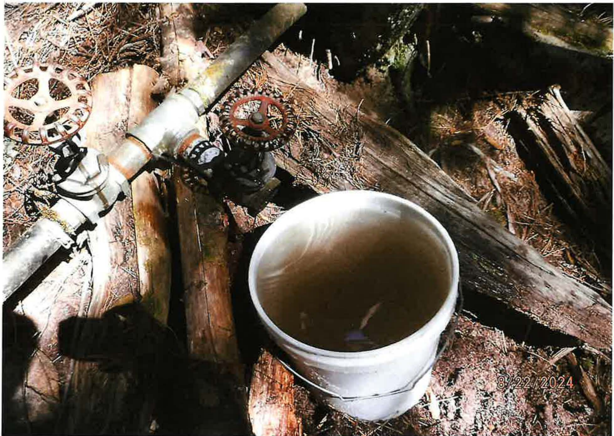
FLOW MEASUREMENTS (3EA) TAKEN FROM 2 ND BLOWOUT VALVE FROM POD
