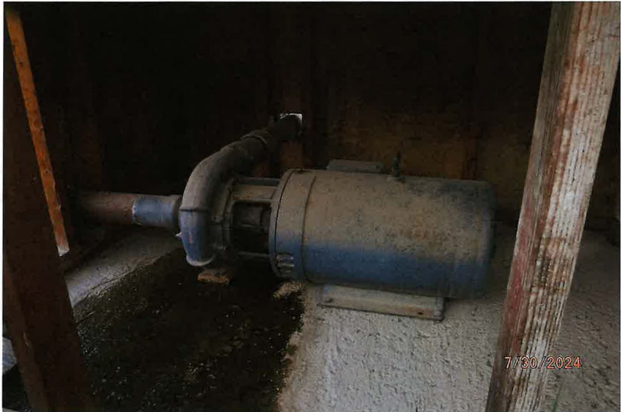
30 HP CENTRIFUGAL PUMP SERVES RIGHT 96-8995 FOR IRRIGATION AND IRRIGATION FROM STORAGE USE; PUMP ALSO SERVES AS A TRANSFER PUMP FOR 96-9901 DRAFTING WATER FROM 24-HR IMPOUNDMENT TO IRRIGATION AT POU.
