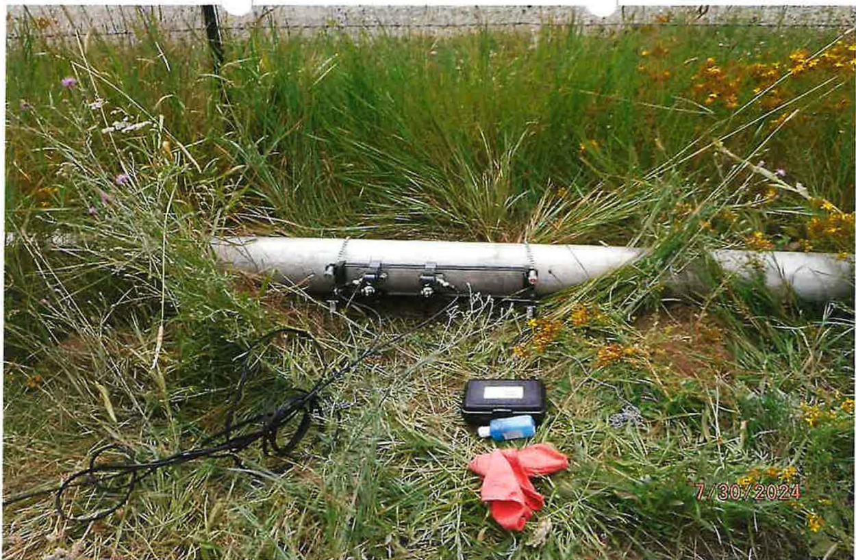
6-INCH ALUMINUM MAIN IRRIGATION TRUNK PIPELINE; CONVEYANCE SYSTEM FOR OVERFLOW WATER FROM 96-9320 TO SERVE 96-9901
