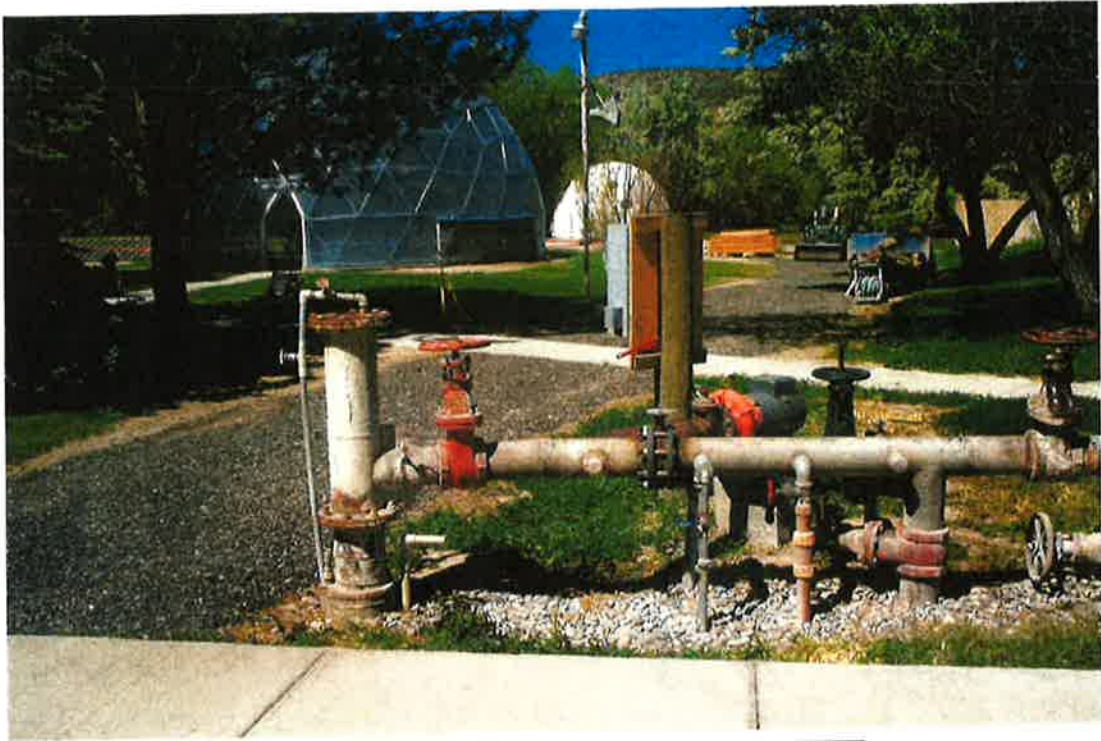
Geothermal Well & Outlets To Various Uses By J E Stanton 6-5-2002 Permit 47-7829
