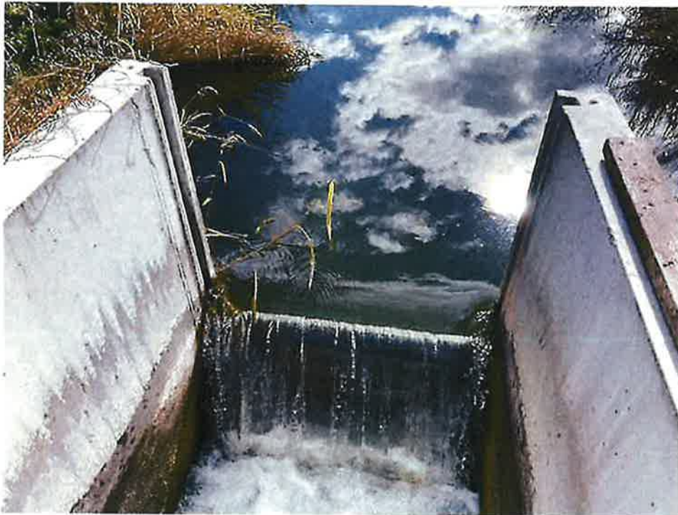
Check structure at head of North Ditch at bifurcation of Upper Haas Ditch. Boards function as a 4-foot suppressed weir
