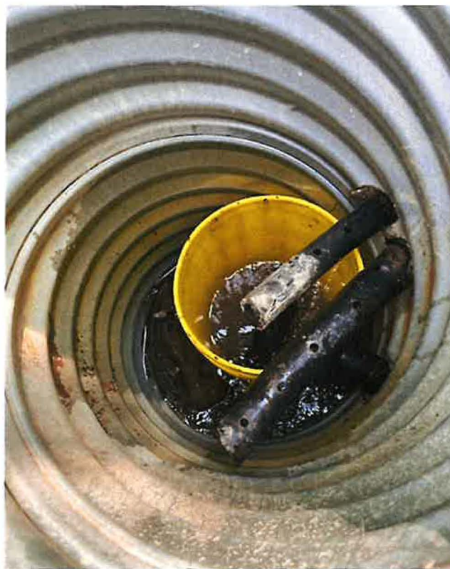
Figure 4: 16" cistern to allow for redirection back to stream. 2" line in bucket carries water to upper pond
