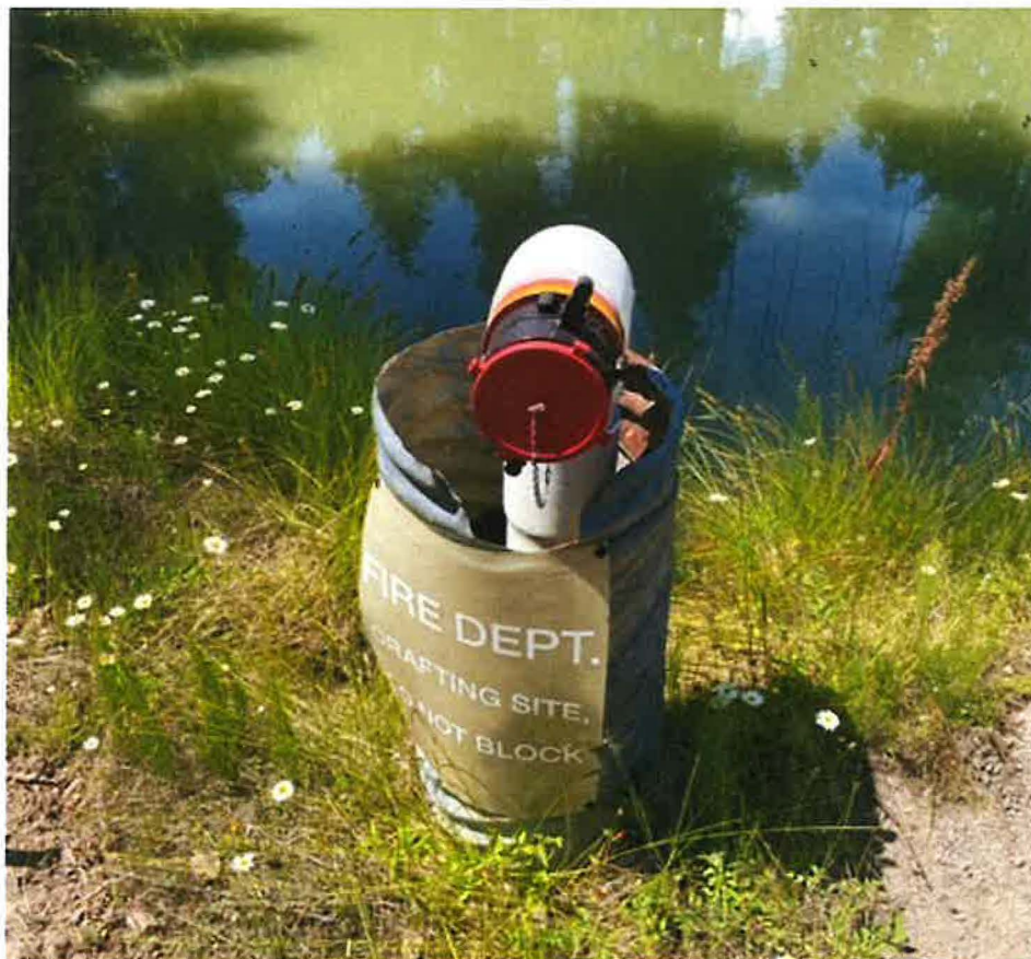
Figure 8: Fire protection hydrant
