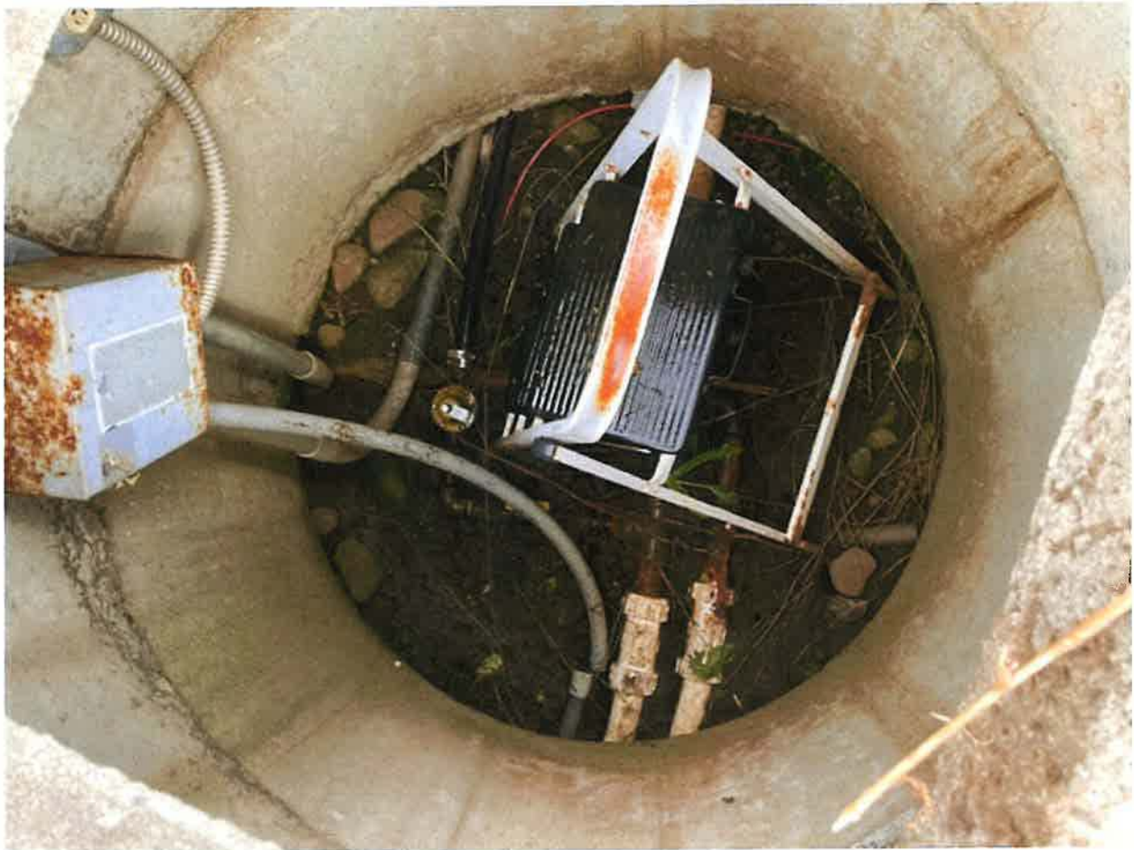
Figure 4: Piping for domestic and irrigation systems next to well
