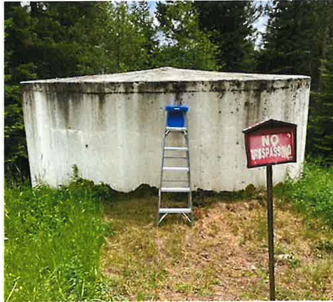
Figure 6: 35,000 gallon storage tank
