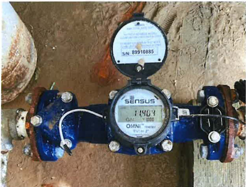
Figure 4: Flow totalizer in pump house
