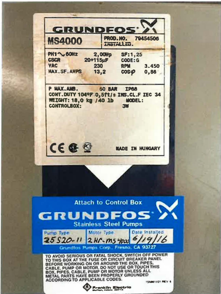
Figure 5: Well pump make/model
