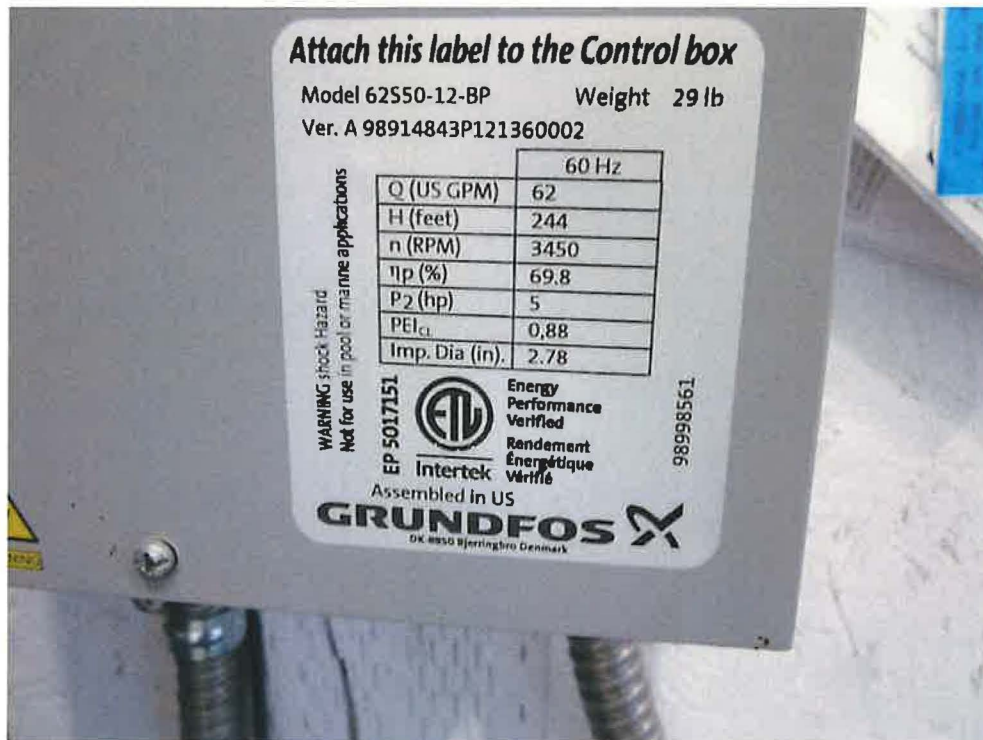
Figure 7. Photograph of pump specifications to the right of the pump control screen two photographs above.
