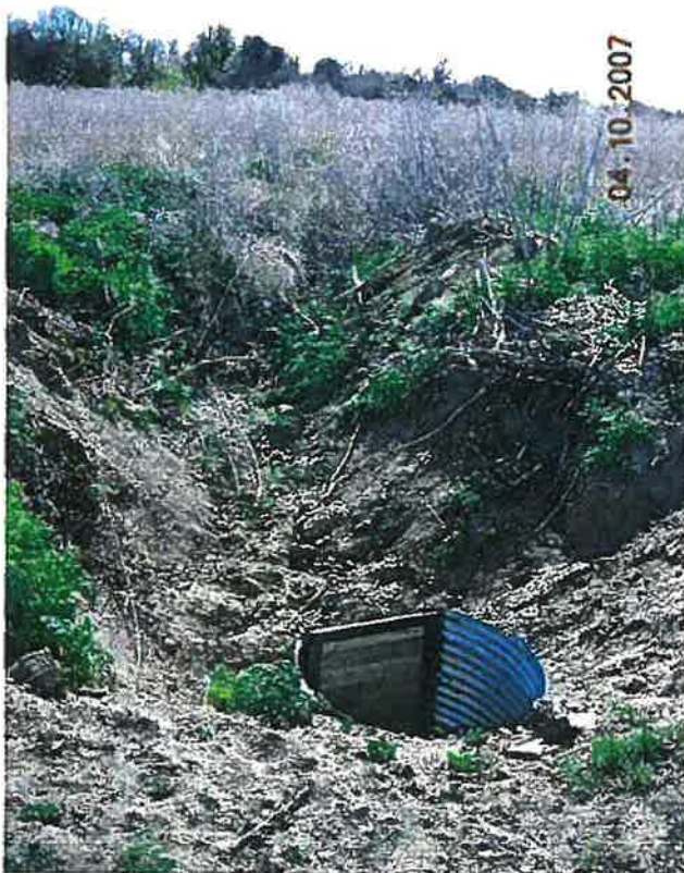
Photo 10: Outlet Structure for East Ponds (63-32460)
