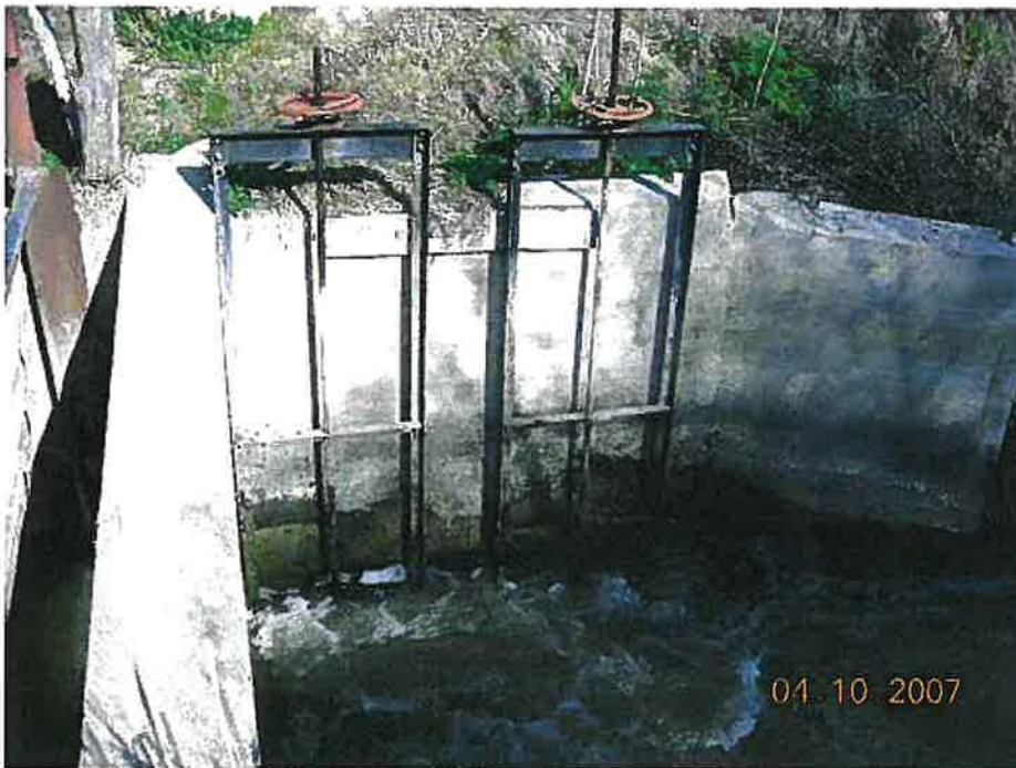
Photo 2: Headgates to the Haas Canal (24-inch)
