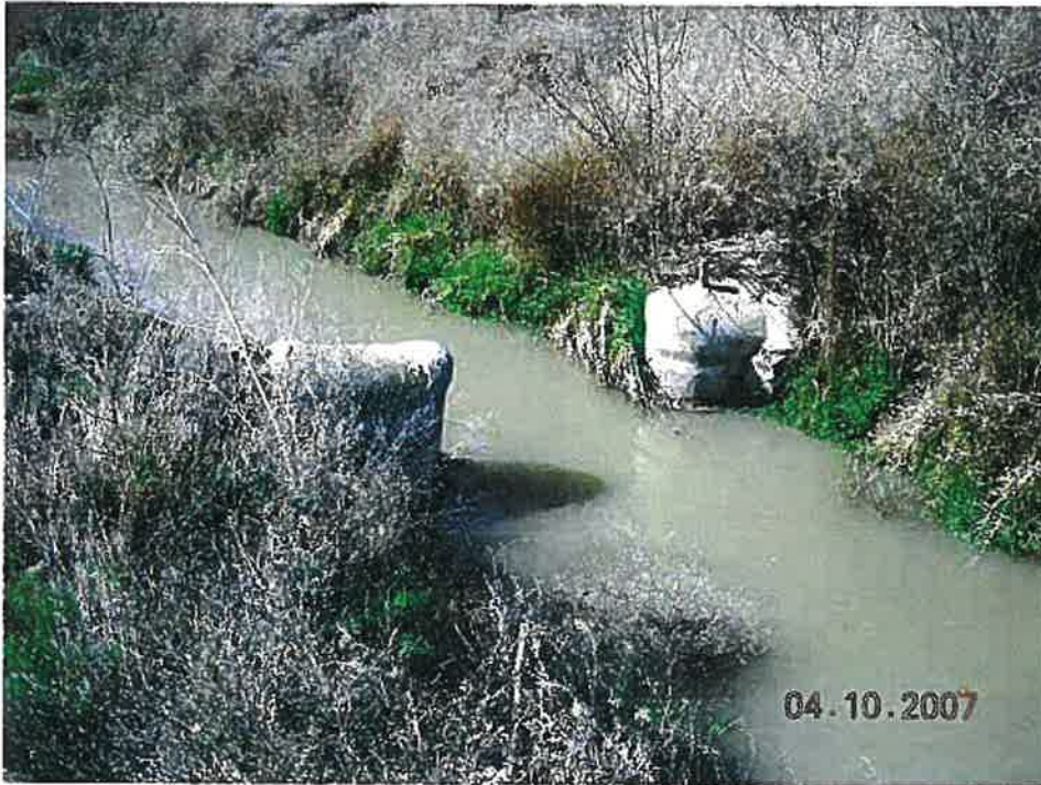
Photo 11: Siphon taking water from ponds across Haas Canal toward East End Drain
