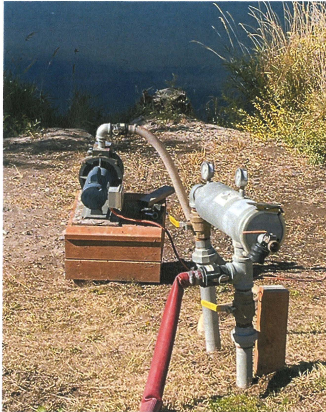
Figure 2 Photo of point of diversion, a 2hp Munro LP Series pump diverting water from the Snake River.
