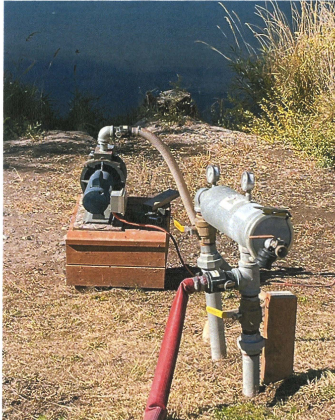
Figure 2 Photo of point of diversion, a 2hp Munro LP Series pump.
