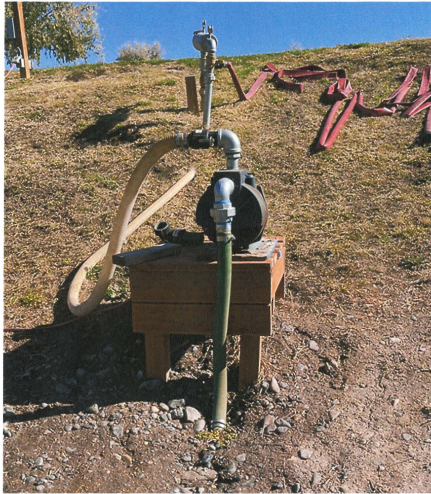
Figure 4 Photo of point of diversion, including buried pipe from river and 2hp pump.
