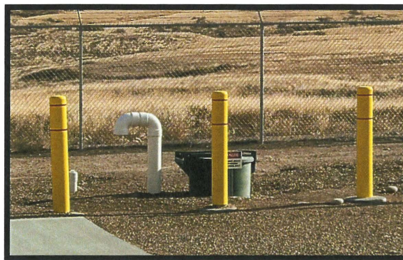
Photo 17b- Hatch and vent for 10,000-Gal storage tank.
