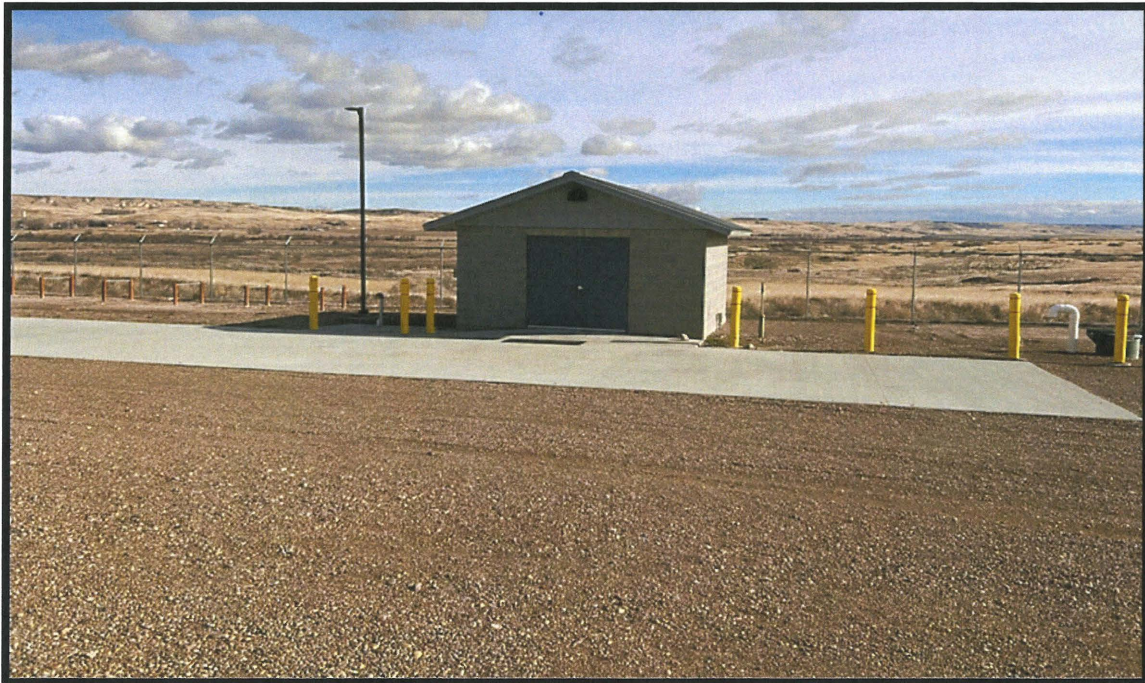
Photo 17a- Truck fill station with the hose hookup riser on the left of the pump house and the green top of the 10,000 Gal storage tank on the right with the white vent next to it.
