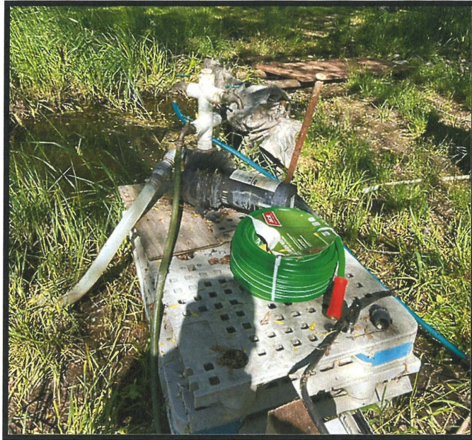
Photo 2- Pump with 1 1/2" PVC manifold distributing to 4 hose bibs.
