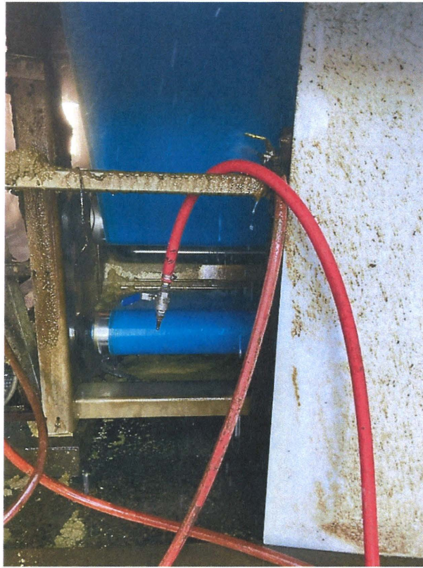
Figure 9 Production belt and two \frac{3}{4} " hoses with Global Industrial CF8M nozzles.
