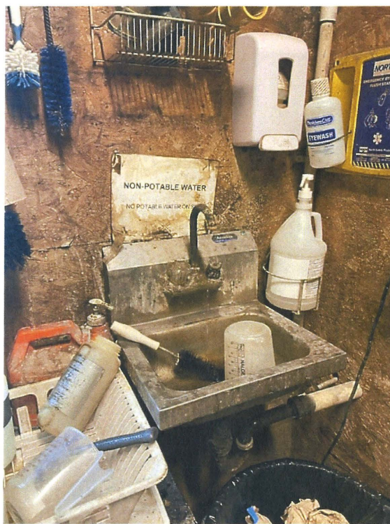
Figure 11 Single hand washing sink, used intermittently.
