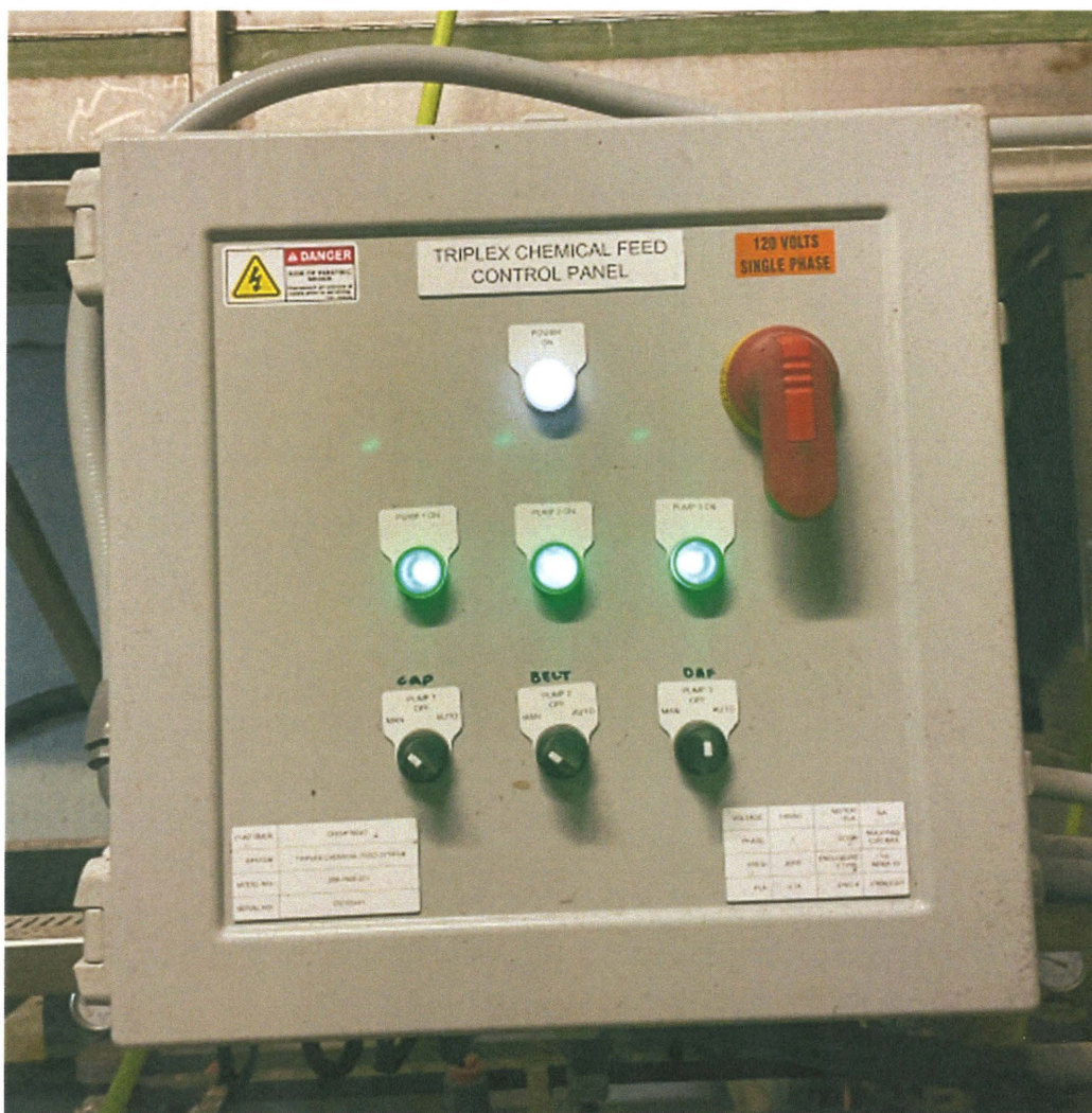
Figure 12 Triplex chemical feed control panel associated with the polymer treatment associated with wastewater system for WR 65-24209.
