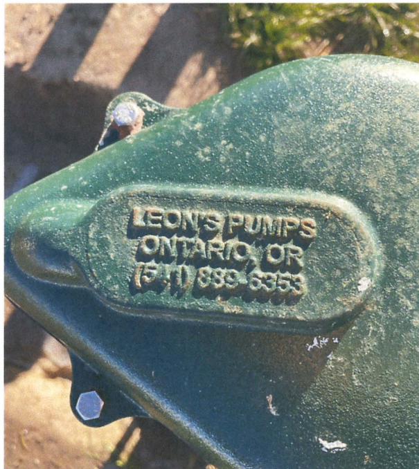
Figure 4 Leon's Pumps Ontario, Oregon tag on well D0104334.
