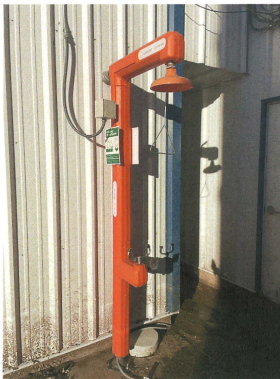
Figure 8 Guardian brand GFR3100 freeze resistant emergency shower and eyewash station. Shower head and eyewash both have 20GPM flow control.
