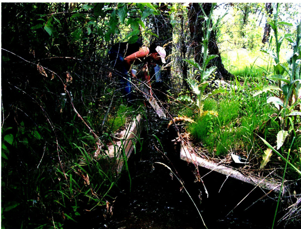
6/25/14 Pine Creek Diversion Inspection: Site #5 "Horse Flat" (Pine Creek) concrete structure potential measuring device in disrepair.
