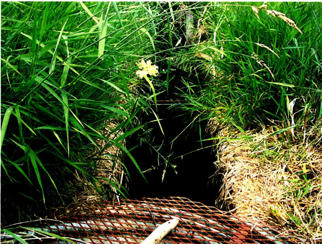
6/25/14 Pine Creek Diversion Inspection: Site #7 "Noah Upper Diversion" (Pine Creek) fish screening structure with no weir blade to allow for measurement.
