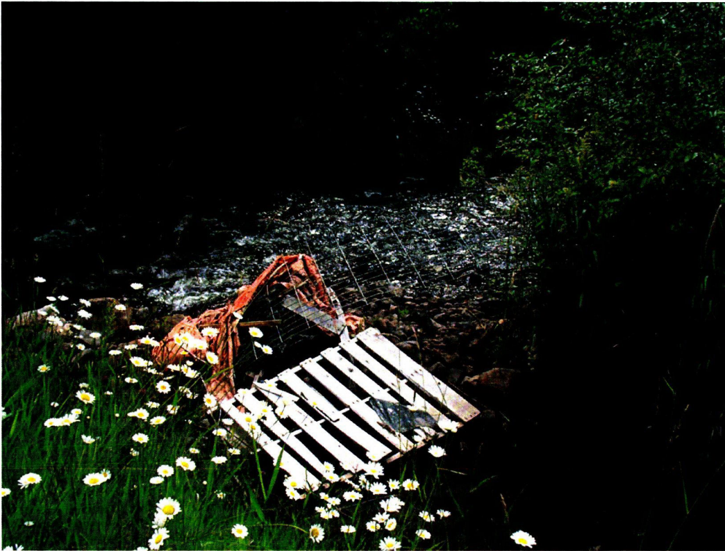
6/25/14 Pine Creek Diversion Inspection: Site #2 "Mink" (Pine Creek) head of diversion ditch off Pine Creek. No headgate in place.
