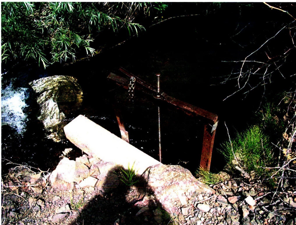
6/25/14 Pine Creek Diversion Inspection: Site #5 "Horse Flat" (Pine Creek) headgate in disrepair.
