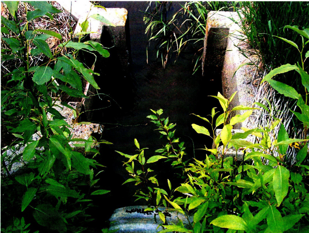
6/25/14 Pine Creek Diversion Inspection: Site #6 "Hansen & Weibe" (Pine Creek) concrete structure potential measuring device in disrepair.
