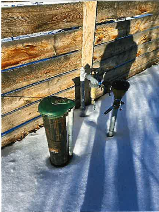
Well D0075978 and irrigation system shut off
