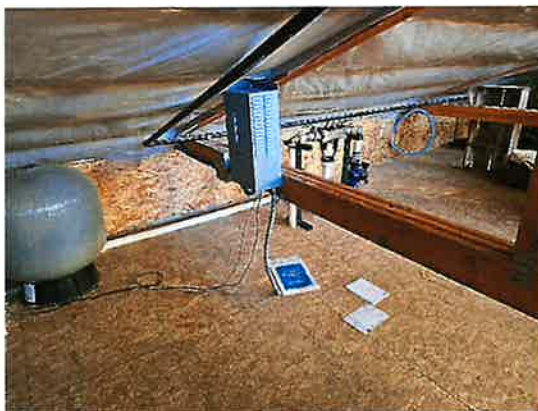
Attic housing flow meter and pressure tanks
