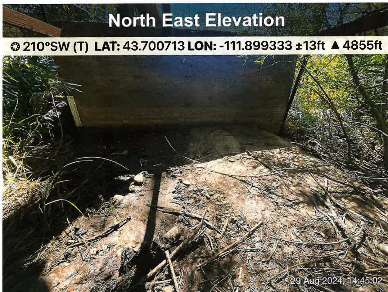
8ft wide weir with high water mark at 0.6 feet above lip of weir.
