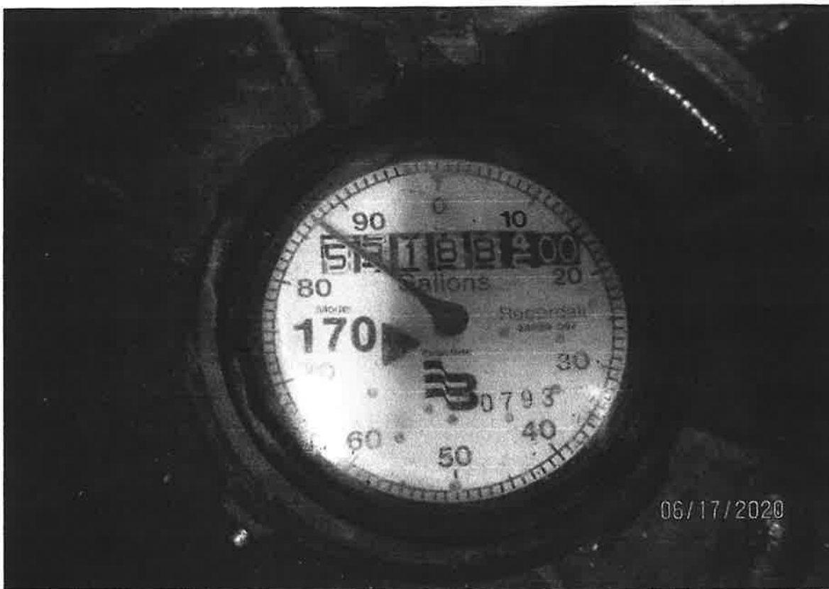
FLOW METER INSTALLED ON SYSTEM
