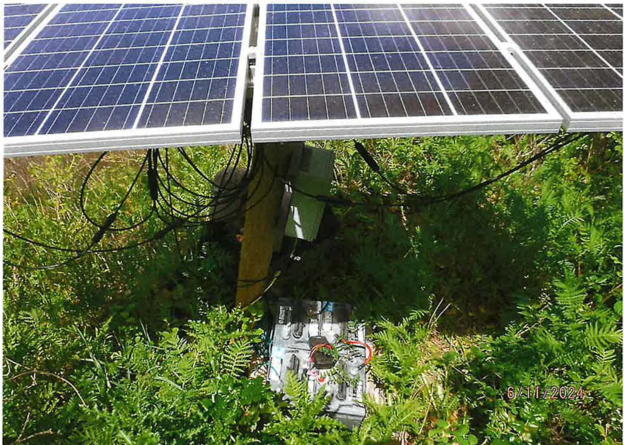
POD – SOLAR PUMP WITH BATTERIES USED FOR SOLAR DIVERTING PUMP
