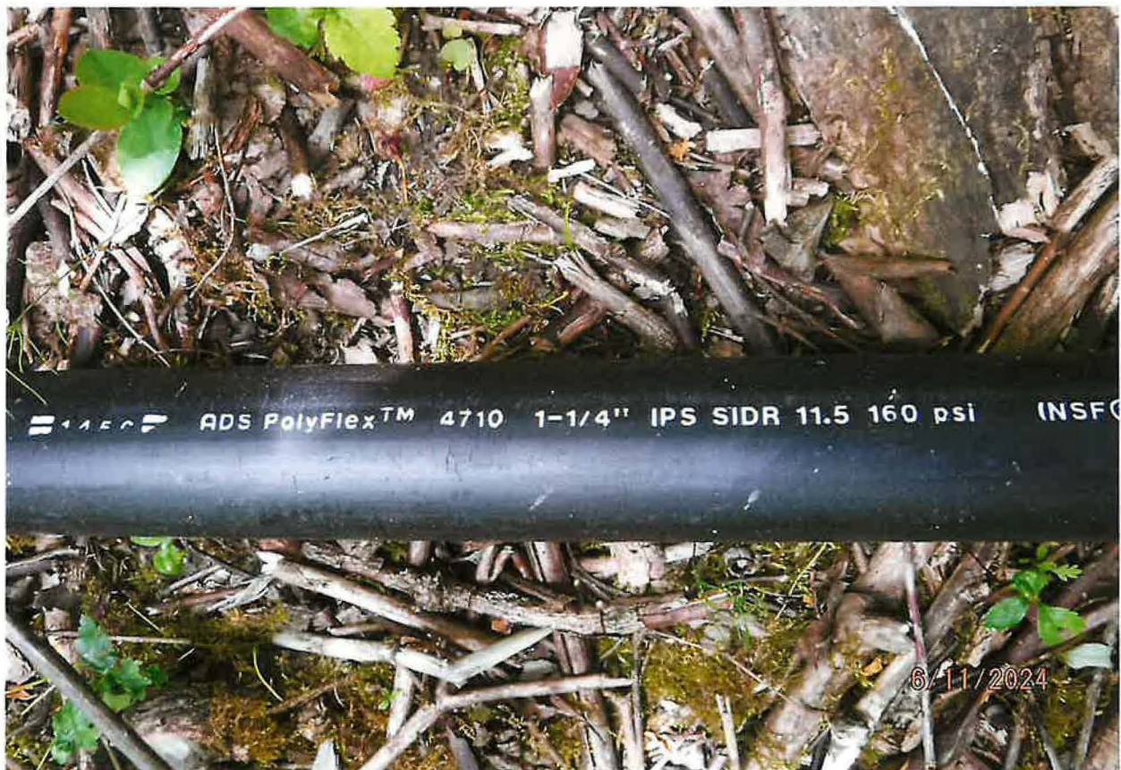
1-1/4 INCH POLYPIPE CONVEYANCE PIPELINE
