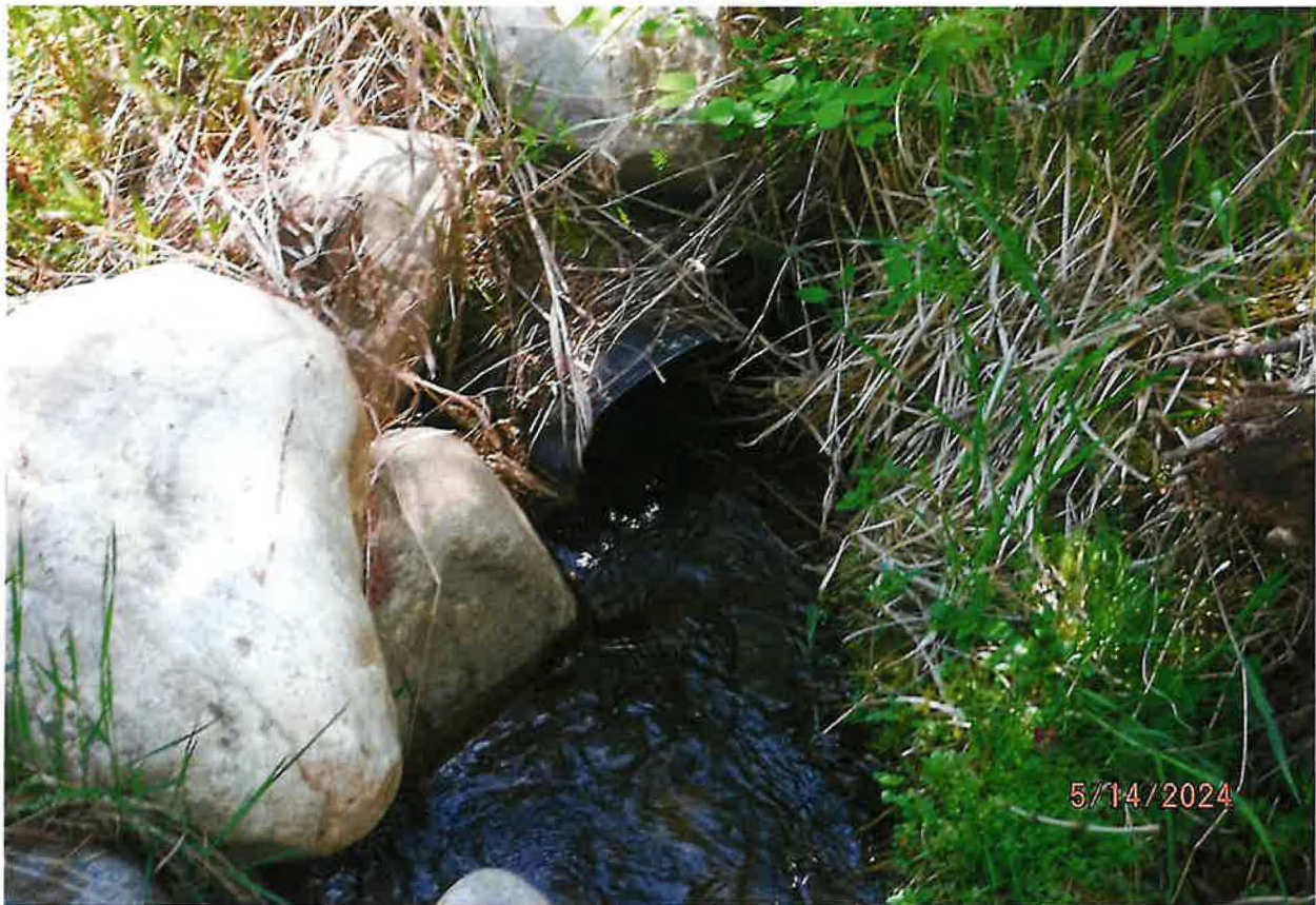
CONVEYANCE DITCH ENTERING POLY PIPE BEFORE INFLOW TO STORAGE POND
