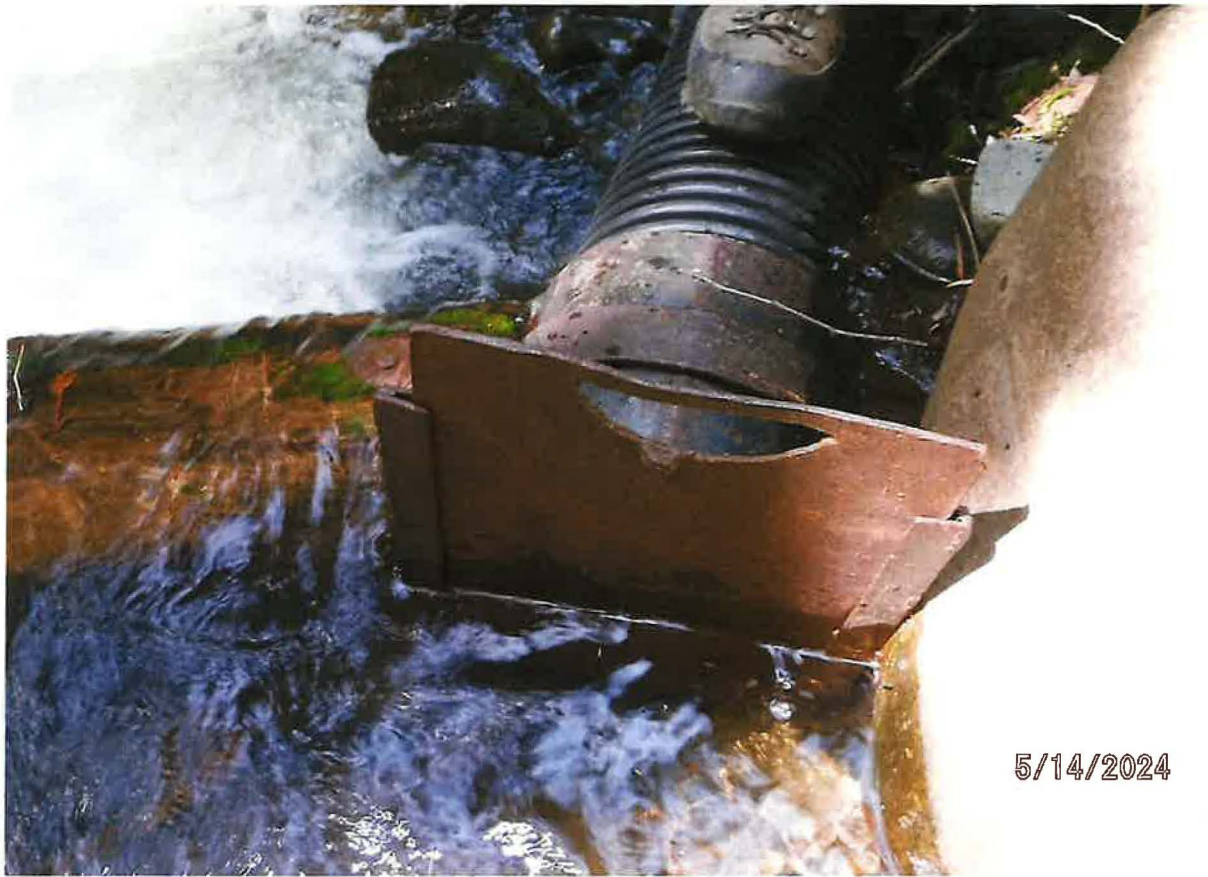
POD – PLATE METAL HEADGATE ON 8-INCH DIVERSION PIPE
