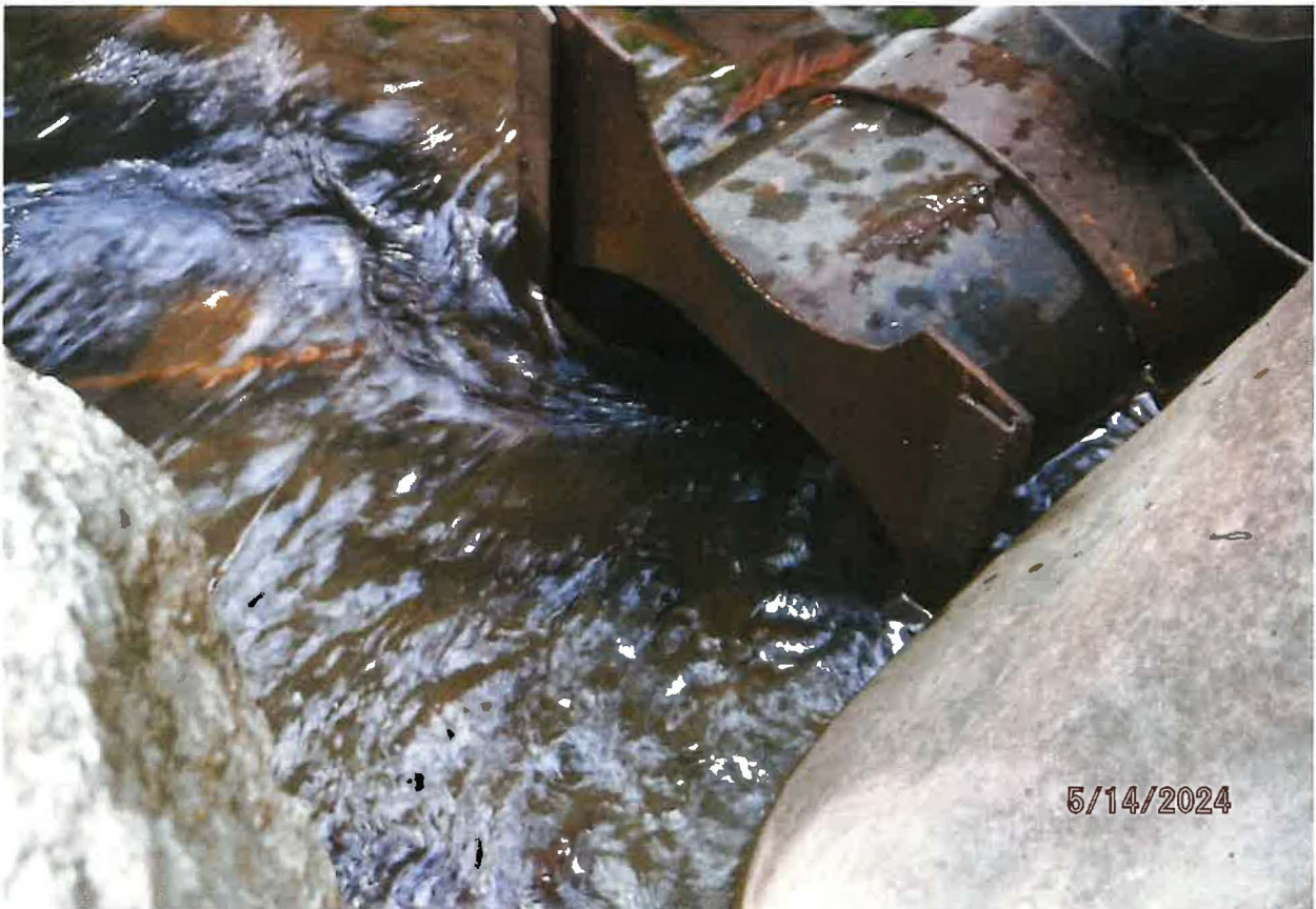
POD – WITH PLATE METAL HEADGATE REMOVED 8-INCH PIPE FILLS TO CAPACITY
