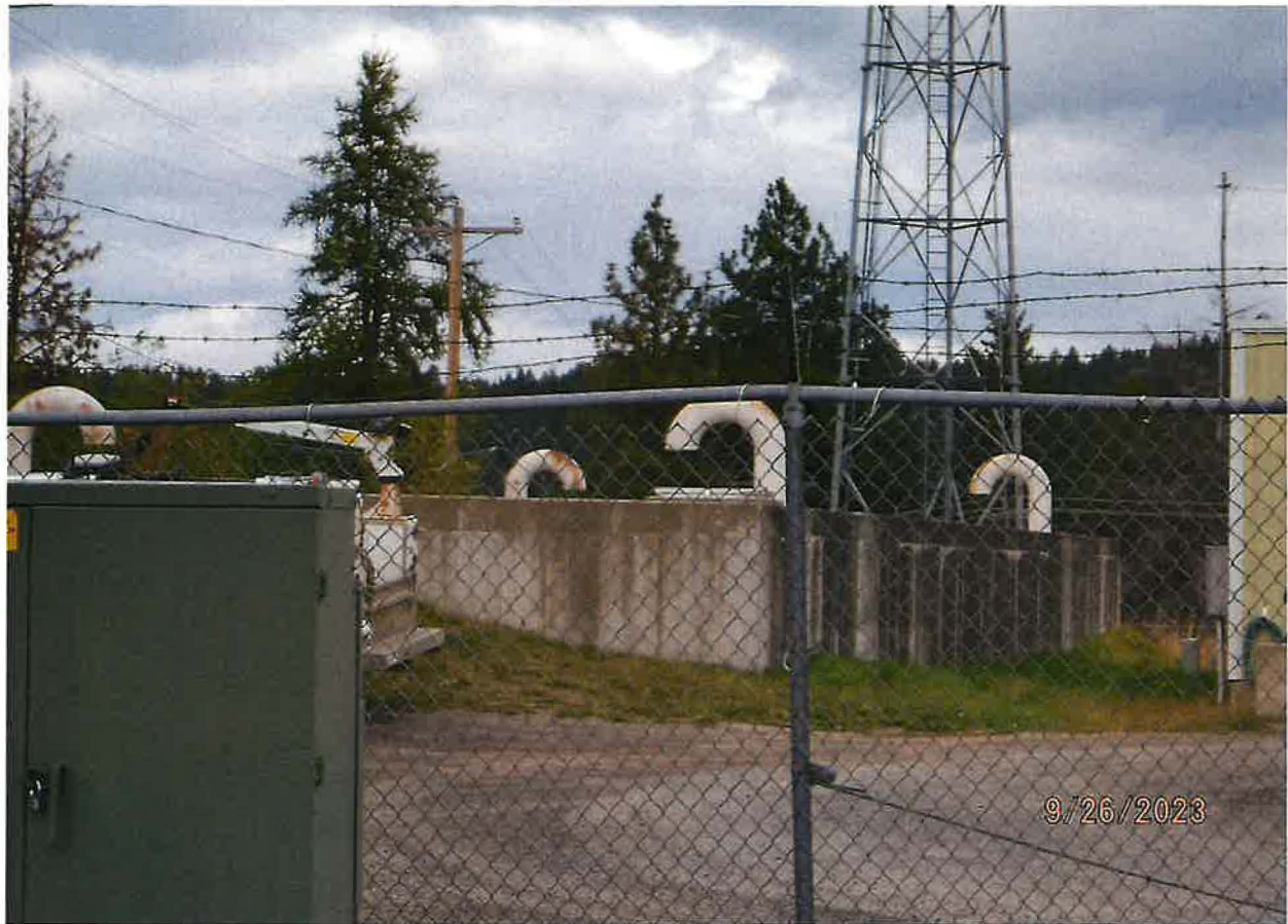
EXAMPLE STORAGE RESERVOIR – 6 TOTAL WITH COMBINED CAPACITY OF 1.7 MIL GALLONS; LOCATED AT PUBLIC WORKS FACILITY
