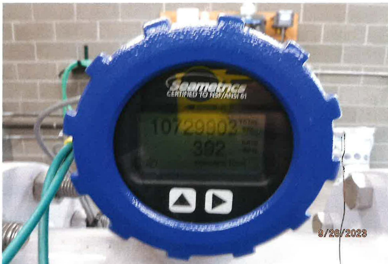
FLOWMETER READING 392 GPM AT CURRENT OPERATING SPECIFICATIONS – PUMPING TO STORAGE RESERVOIR LOCATED “UP-TOWN”
