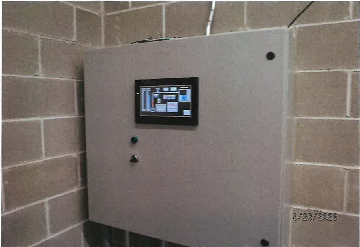
SCADA SYSTEM CONTROL PANEL
