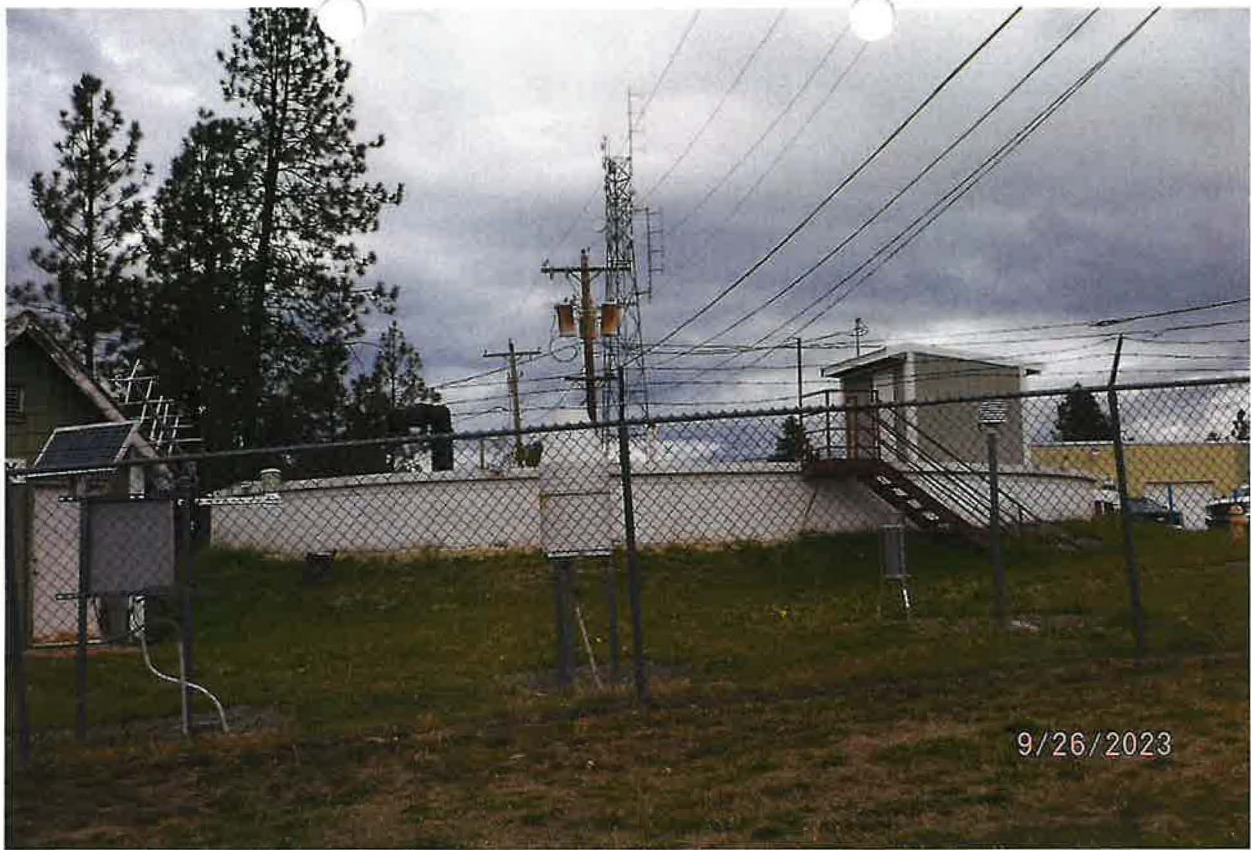
EXAMPLE 1 OF 6 STORAGE RESERVOIRS LOCATED UP HILL FROM WELL PUMP STATION
