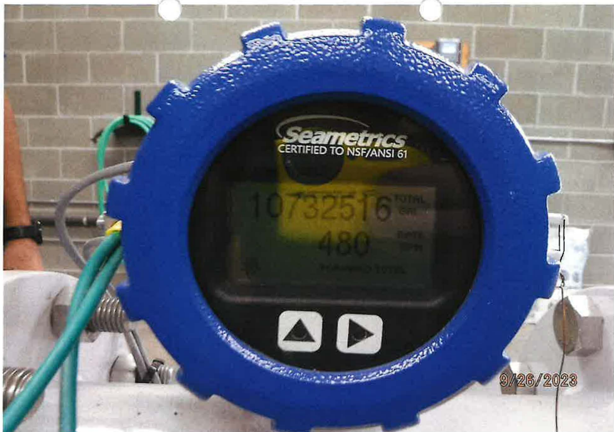
PUMP MOTOR ON WITH FIRE HYDRANT AT PUMP STATION FULL OPEN RESULTED IN 480 GPM – SETTING THAT CAN BE USED TO DISTRIBUTE WATER DIRECTLY TO THE “DOWN-TOWN” PORTION OF WATER SYSTEM
