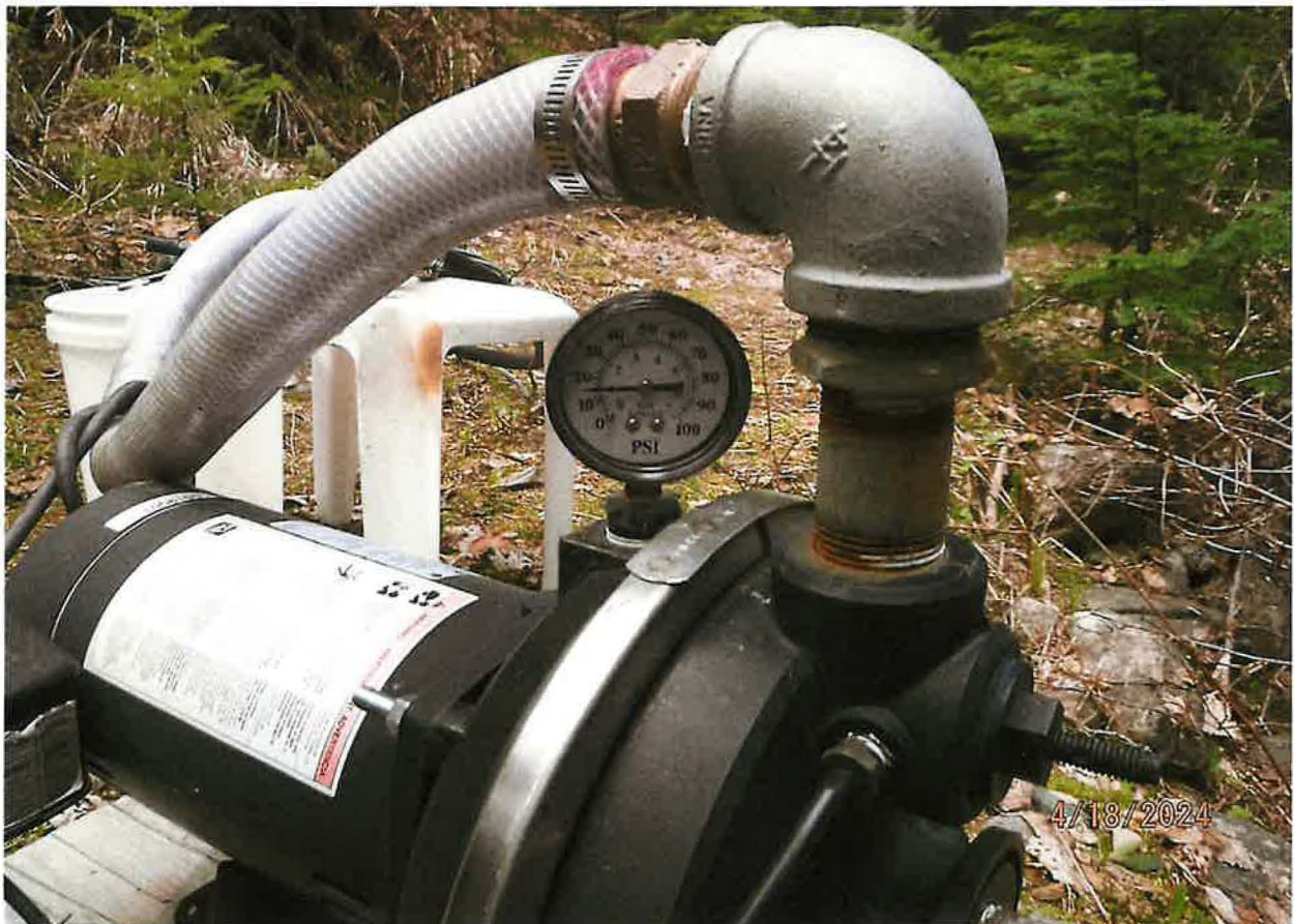
PUMP OPERATES AT 15 PSI
