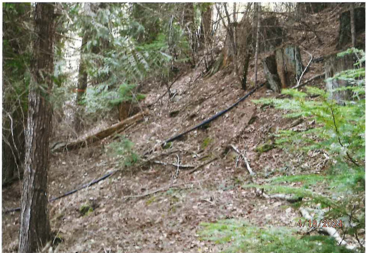
DIVERSION TO STORAGE USE – 1-INCH POLY PIPE ROUTED THROUGH WOODS TO STORAGE POND
