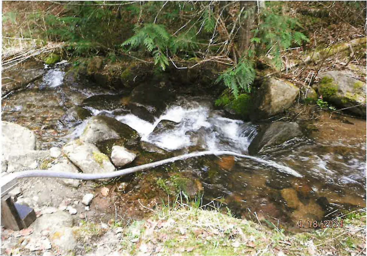
POD – SCREENED FLEX PIPE IN CREEK TO PUMP
