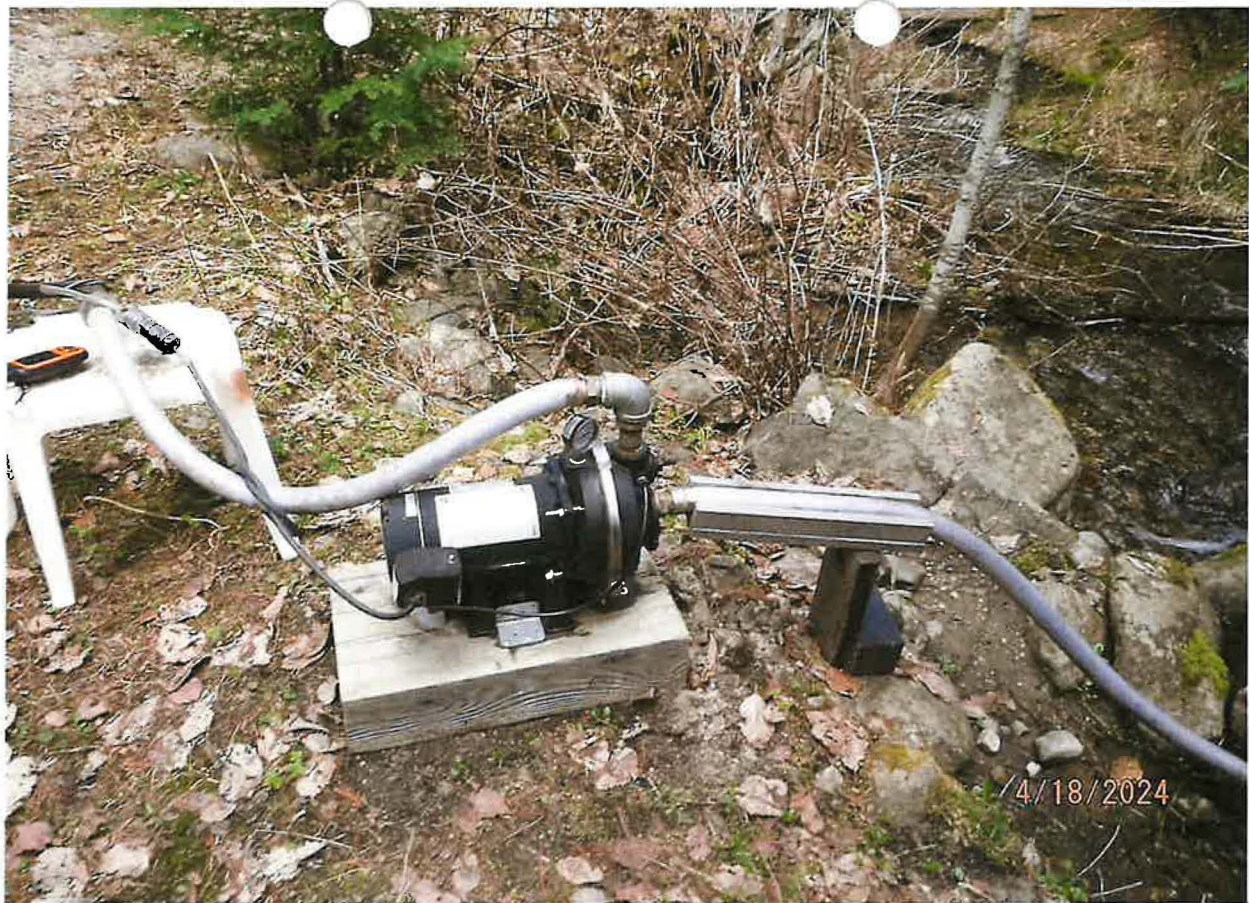
DIVERSION TO STORAGE USE – CONVEYANCE SYSTEM INCORPORATES A 1-INCH DISCHARGE FROM PIPE TO 300-FT OF 1-INCH POLY PIPE ROUTED FROM CREEK TO UPPER POND INFLOW
