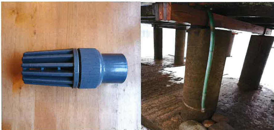
Photos 1 & 2- Intake screen (left) installed on 1" intake line on dock pier (right).
