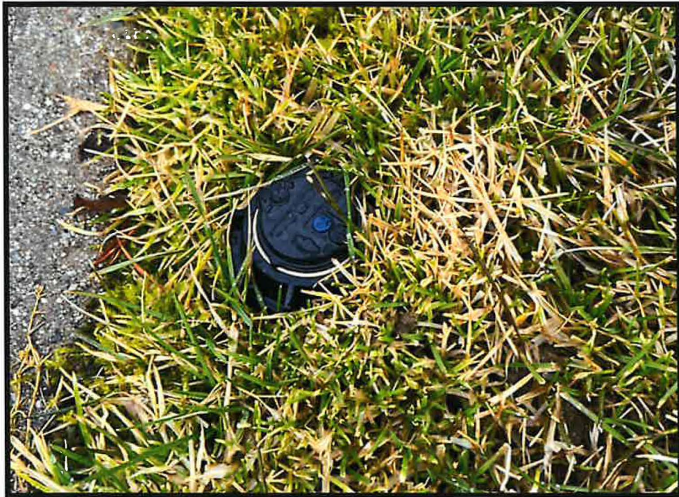
Photo 3- Sprinkler heads used throughout the POU.
