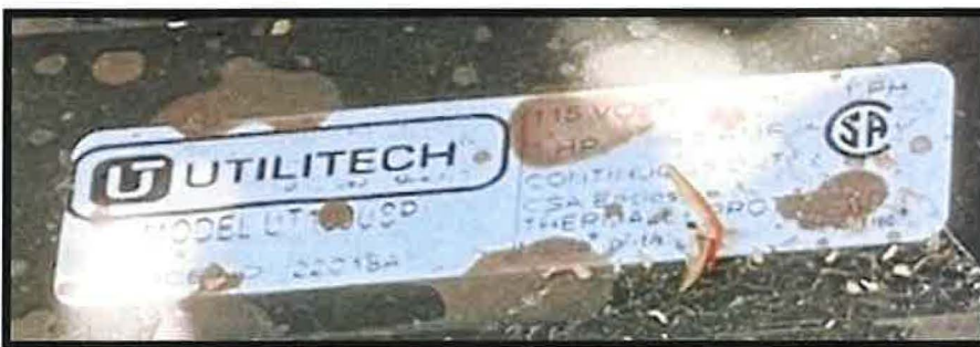
Photo 2-(below) Specification tag on pump.
