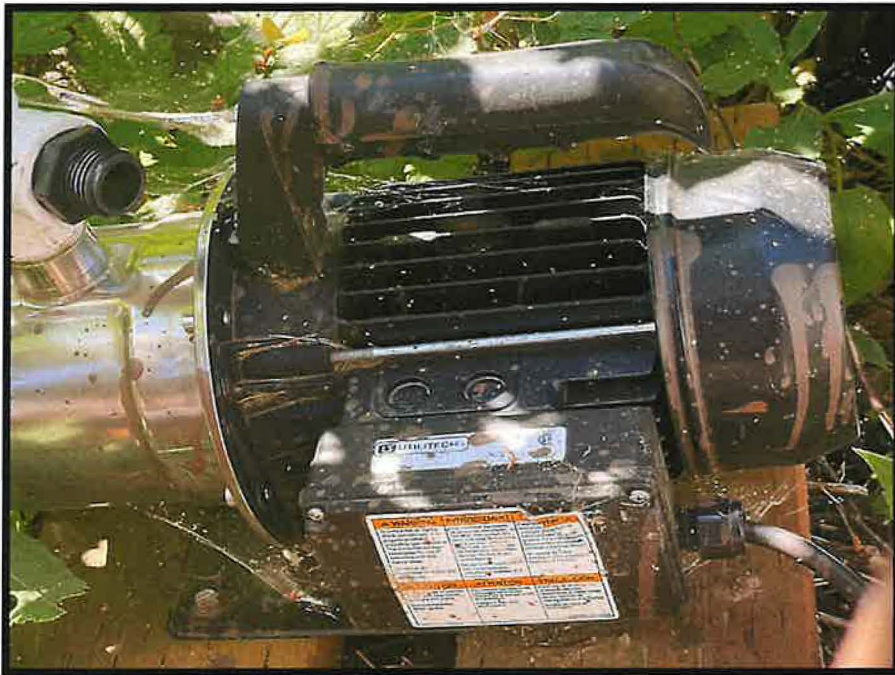
Photo 1- (above) 1 Hp pump with hose bib visible in the upper left of image.
