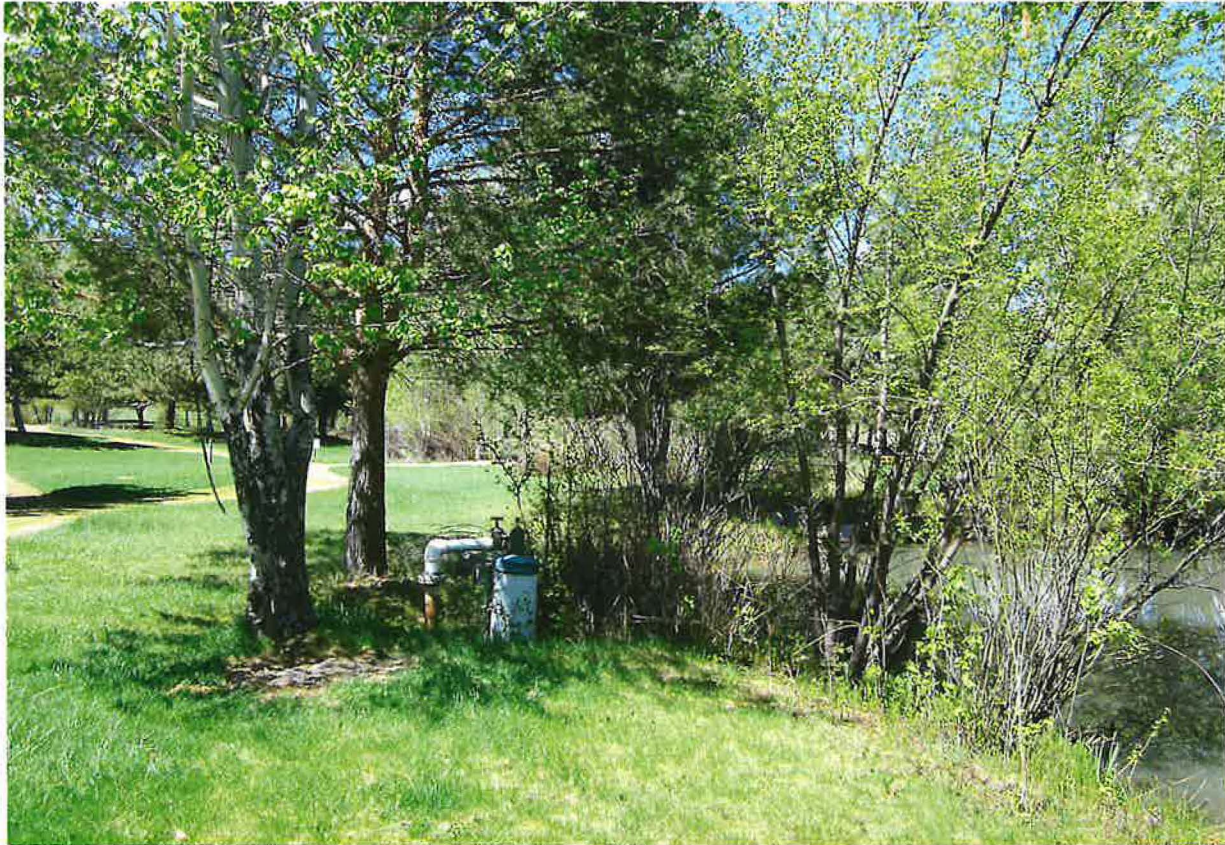
Photo 10- 5 Hp Recirculation pump (no longer functional) located on the south side of the eastern pond. Pump was used to recirculate water from the eastern pond to the western pond to be gravity fed back through the ditch running between the ponds.
