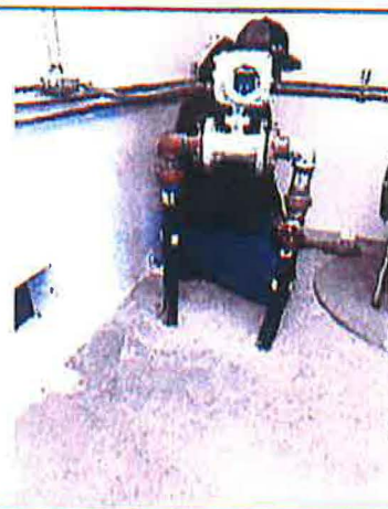
Photo 2: Well flow meter inside the pump house
