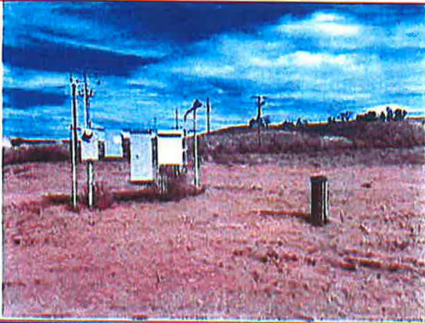
Photo 1: Supply well, pump controls, and power.
