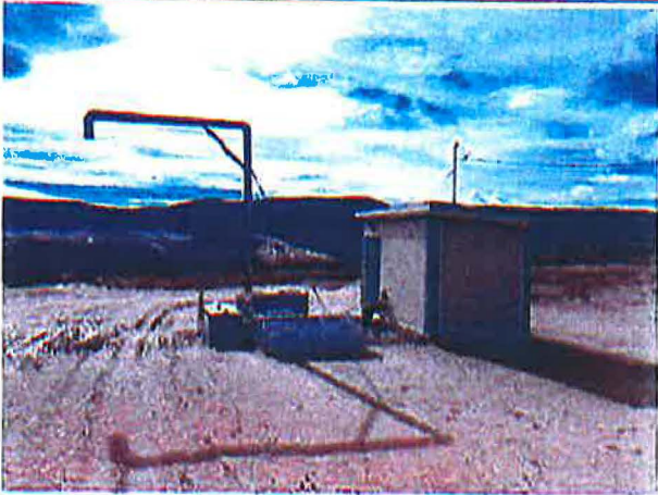
Photo 3: Pump house for PBSL dust suppression system
