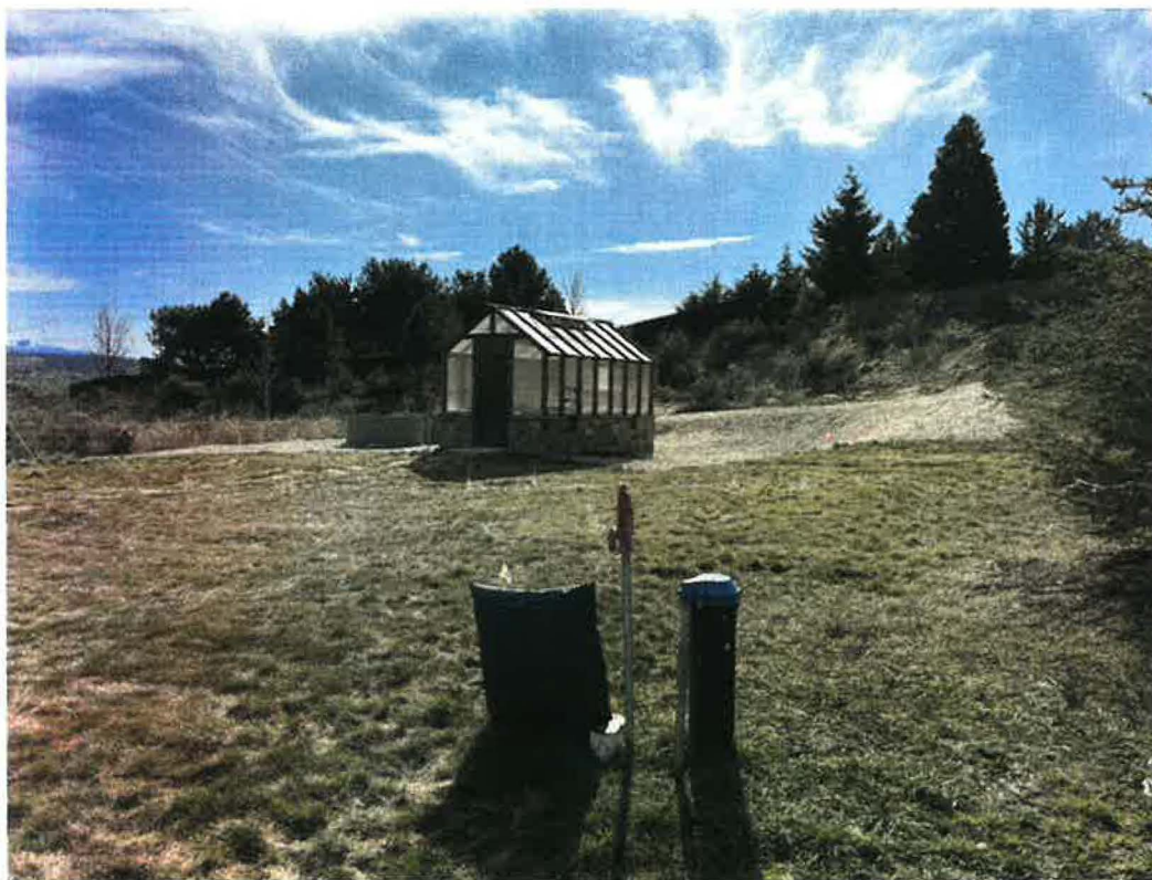
Pump wellhead south of house.
