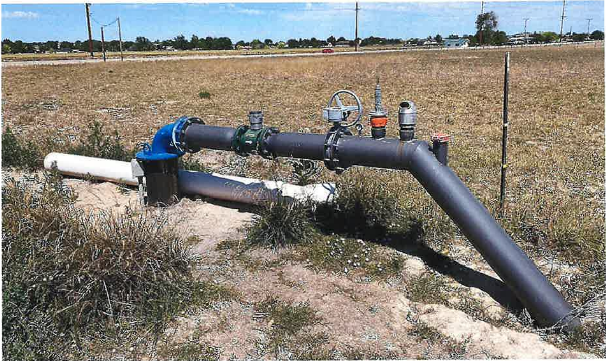
Well and discharge piping.
