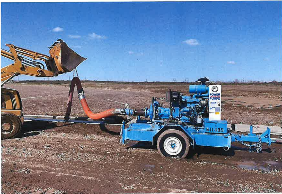
Portable pump at southwest corner of field 4 to pump water to fields 5 and 23
