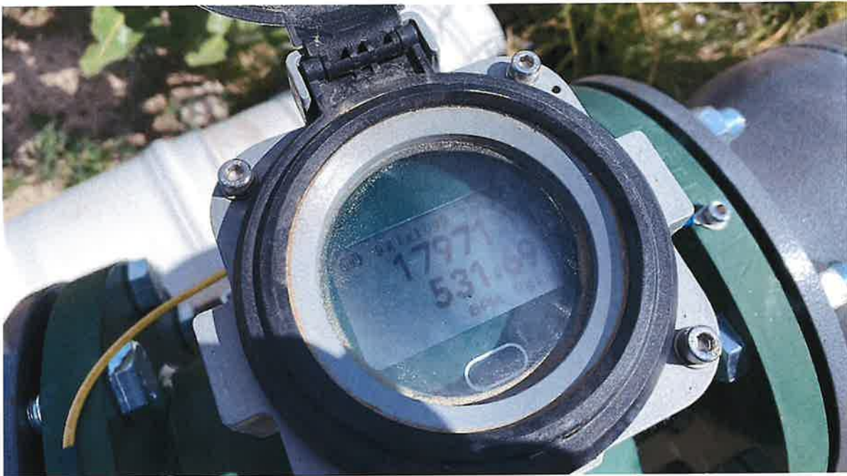
Flow meter display. 531.69 gpm = 1.18 cfs
