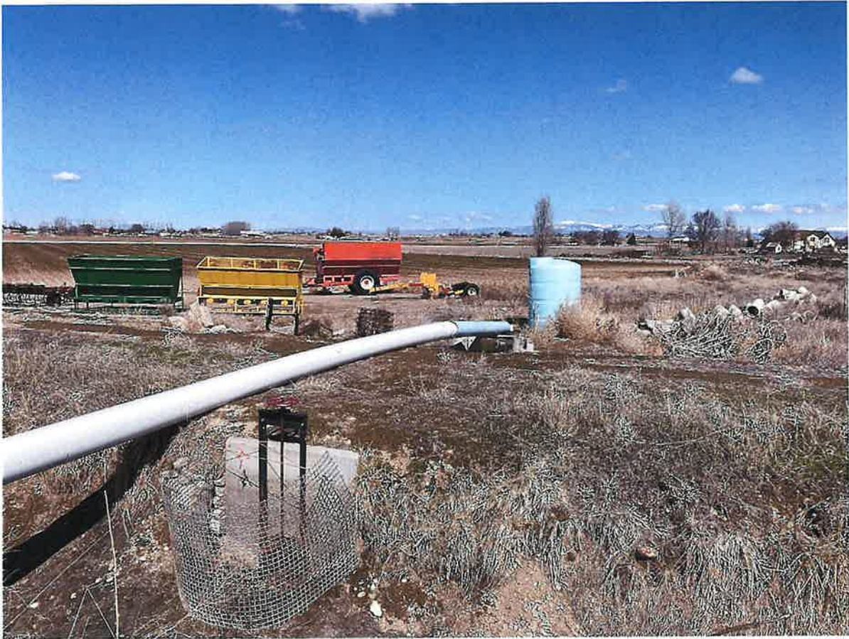
Delivery to field 23 headgate.
