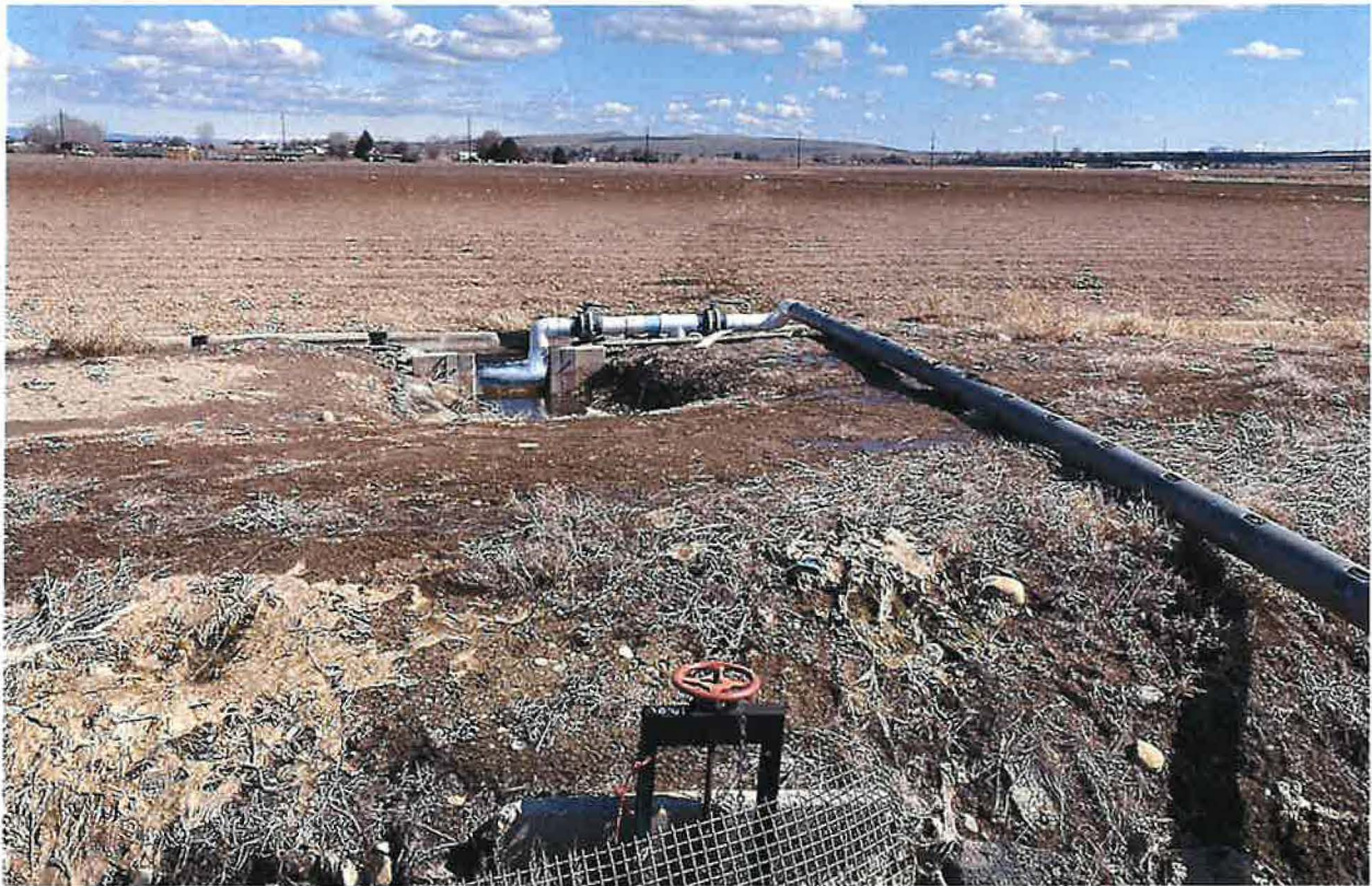
West headbox equipped with pipe to deliver water to fields 16 and 17
