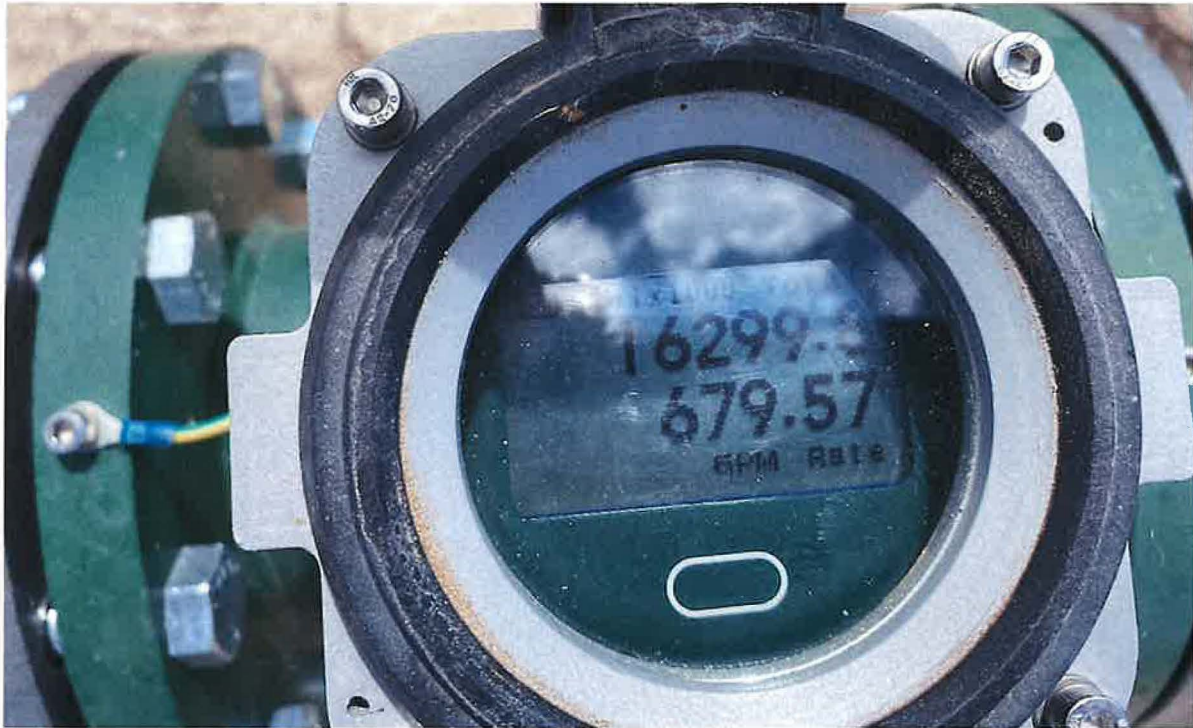
Flow meter display – 679.57 gpm = 1.52 cfs
