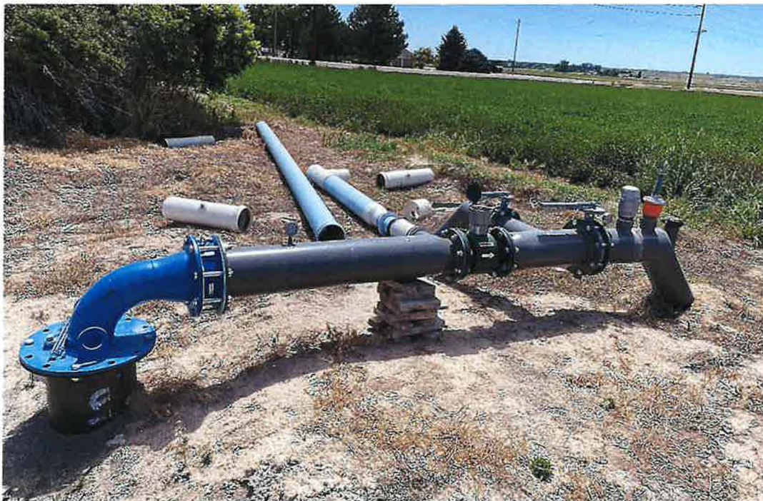
Well head, flow meter, and mechanical pipe.
