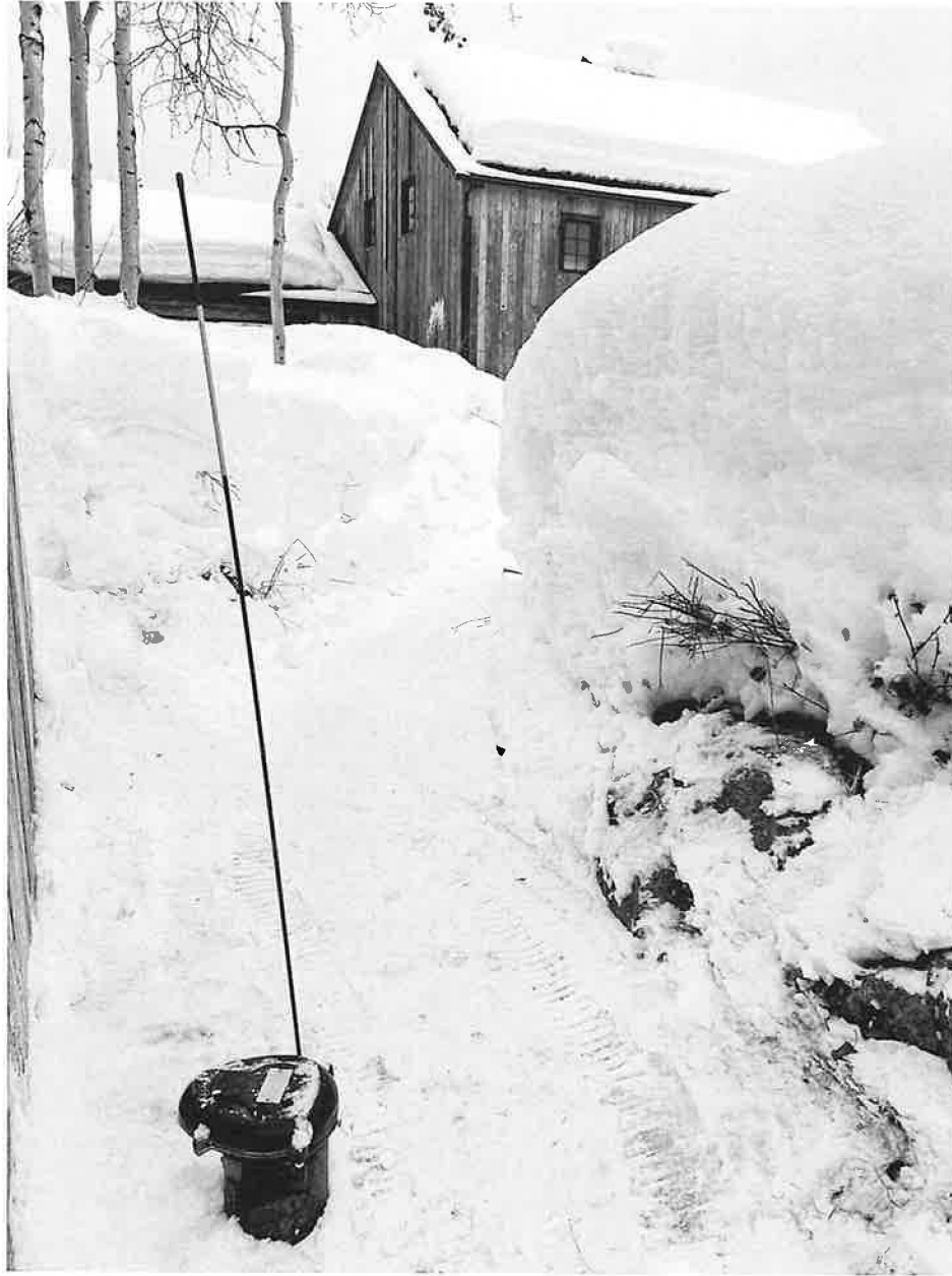
Figure 1: Injection Well on South Side of Residence.
