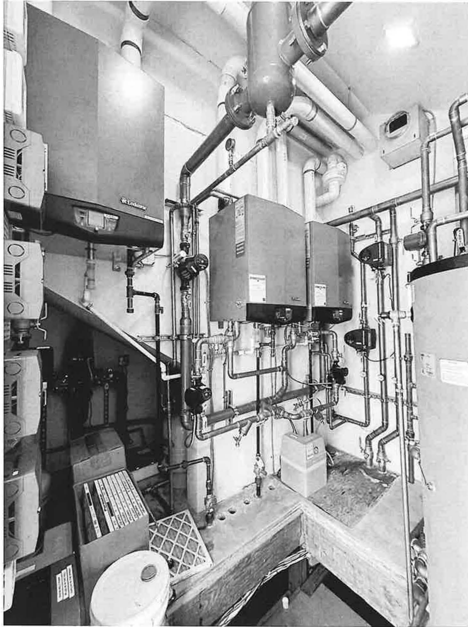
Figure 2: Lochinvar Boiler Units 1, 2 and 3.
