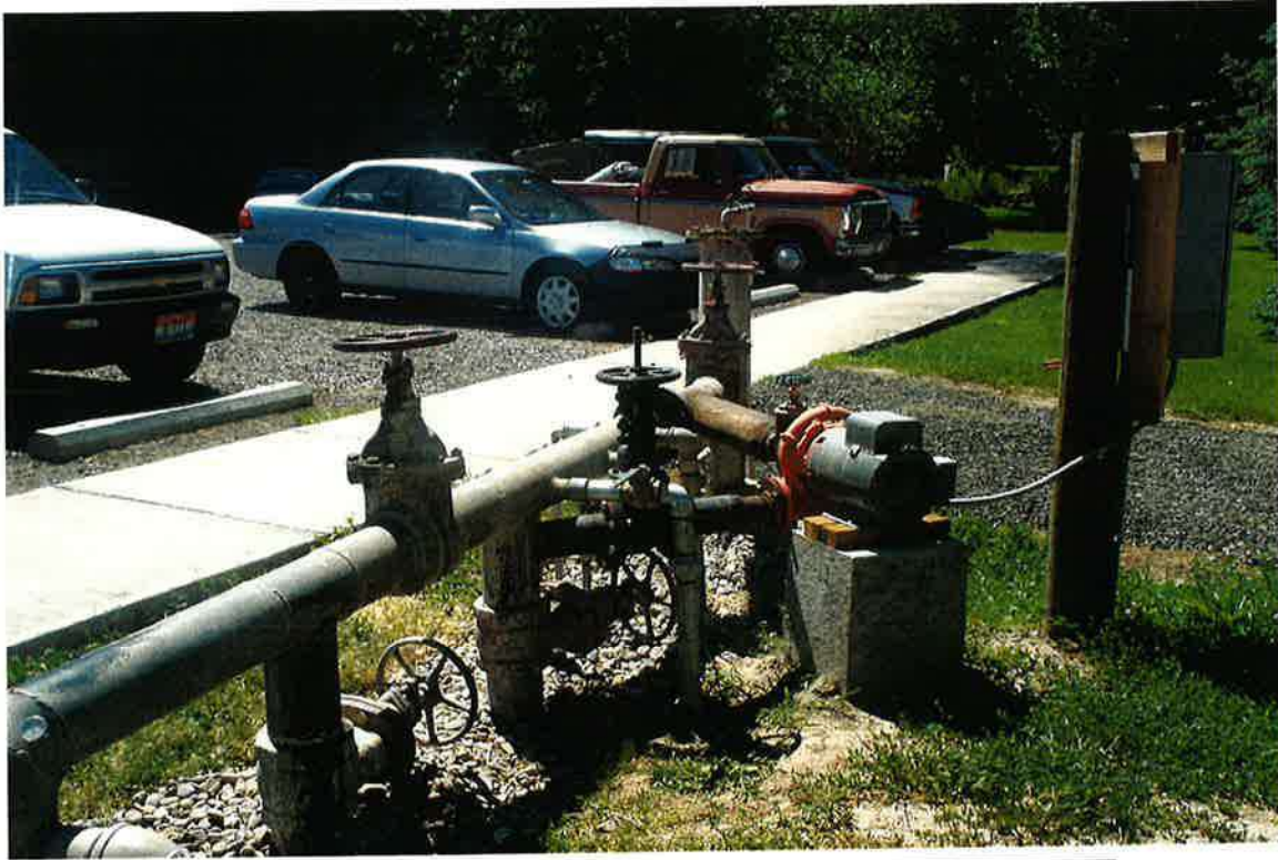
Geothermal Well, Pump For Additional Pressure Looking NE By J E Stanton 6-5-2002 Permit 47-7829 S
