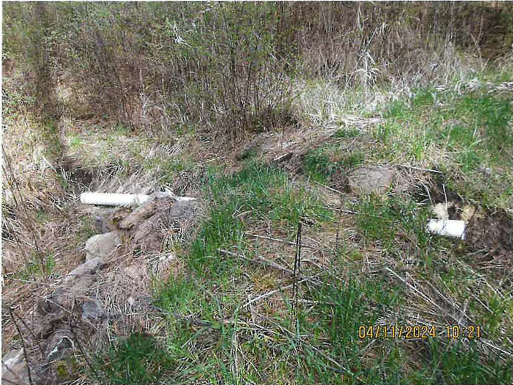
DAM WITH 2 INCH OUTFLOW PIPE TO UNNAMED STREAM
