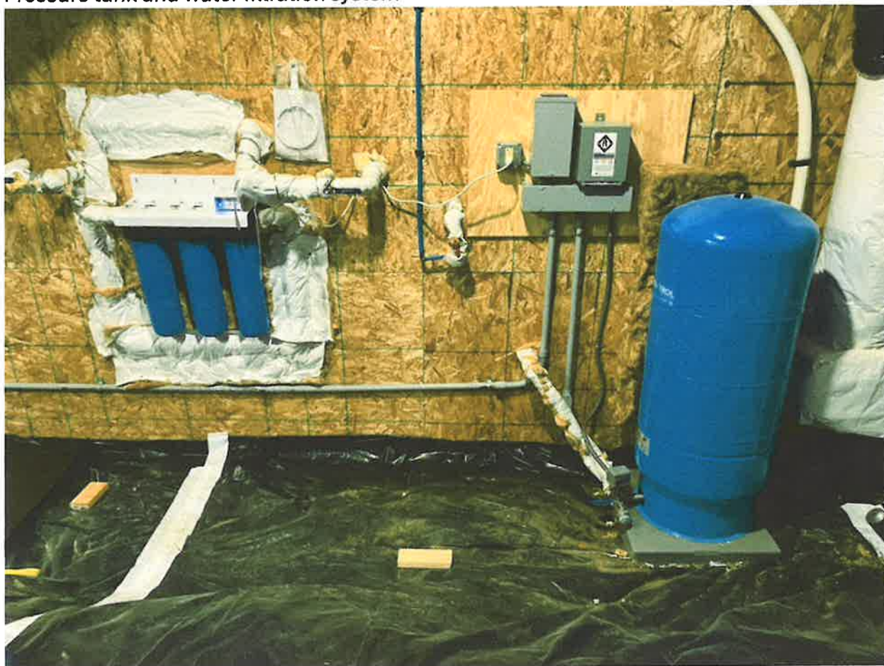
Pressure tank and water filtration system
