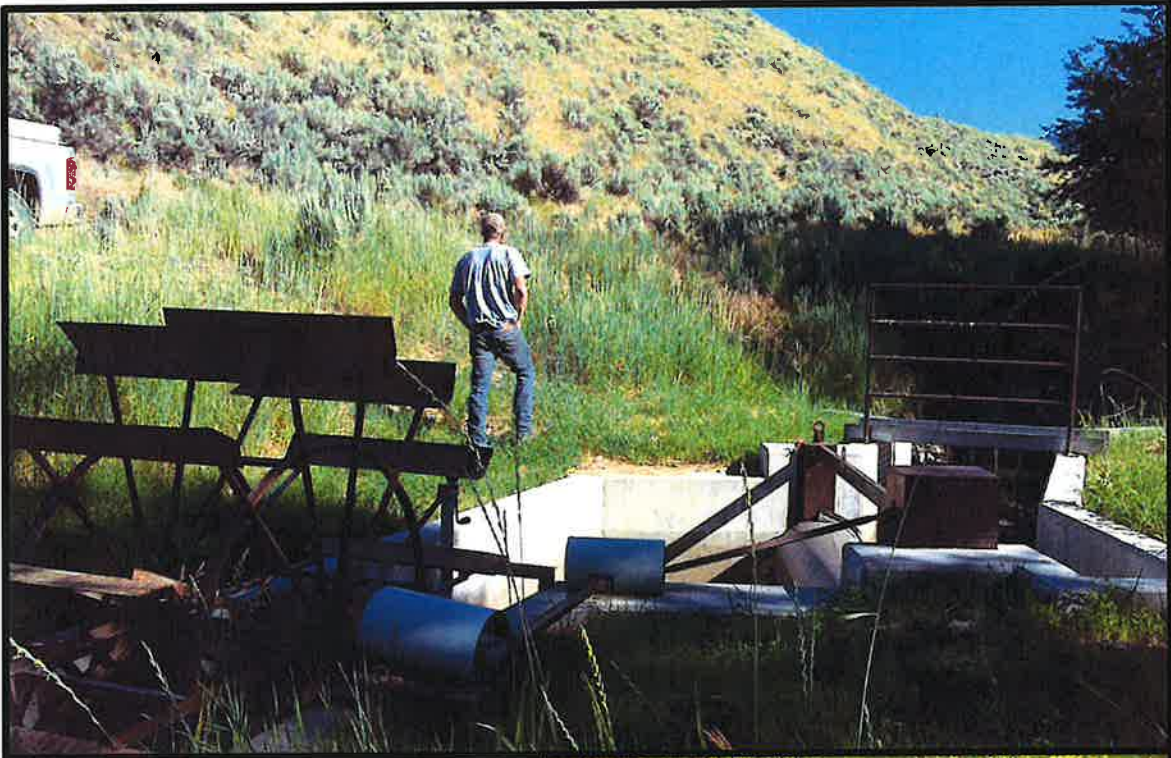
Fish screen with bypass pipe flow (.80 cfs) returning to Bohannon Creek.
