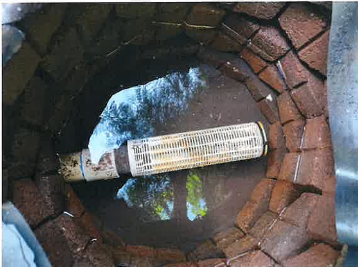
Water Cistern, Water Intake and 2" PVC Water Pipe
