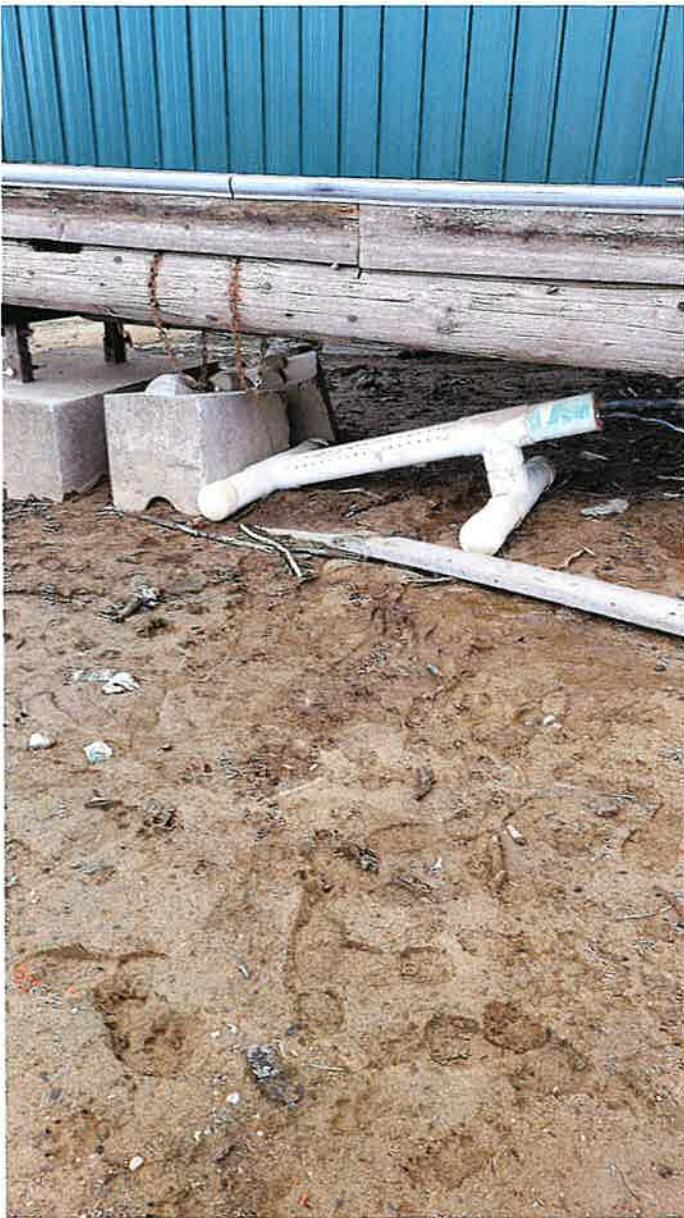
Picture of pump cradle underneath dock
