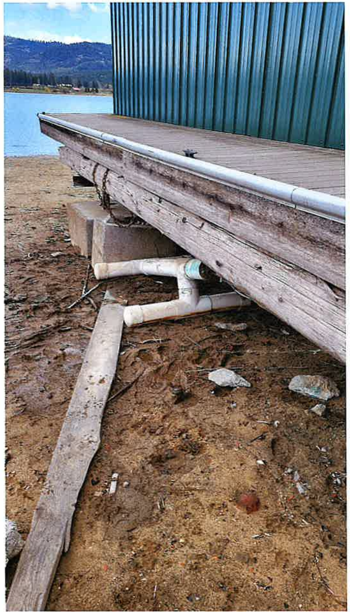
Pump cradle underneath dock - Facing the river
