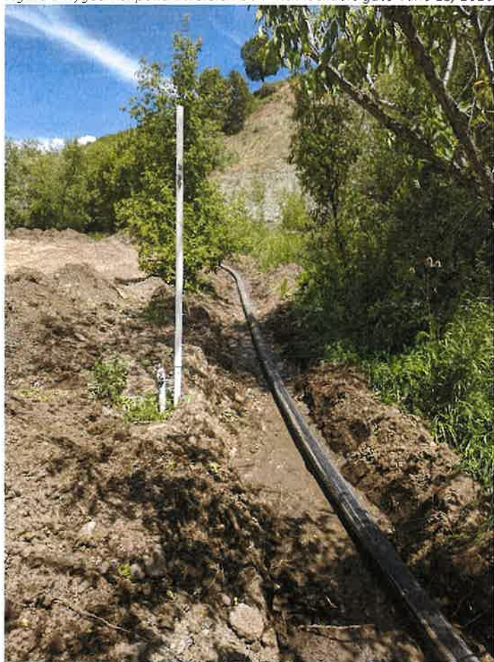
Figure 4 Hygee Fish Pond 6" Line South of Cabin June 18, 2020
