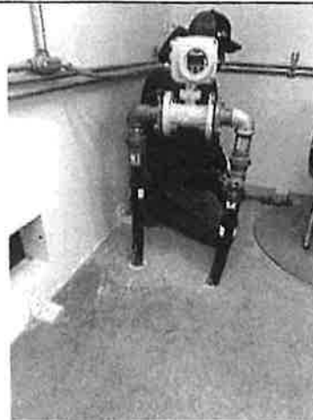
Photo 2: Well flow meter inside the pump house
