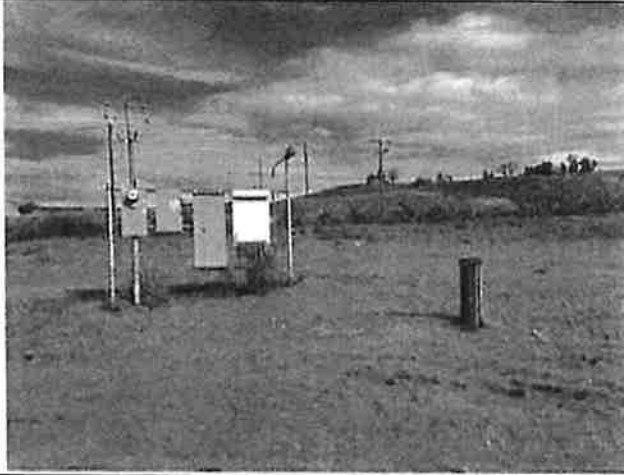
Photo 1: Supply well, pump controls, and power.
