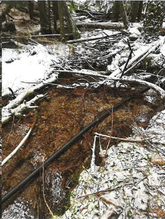
main water line
