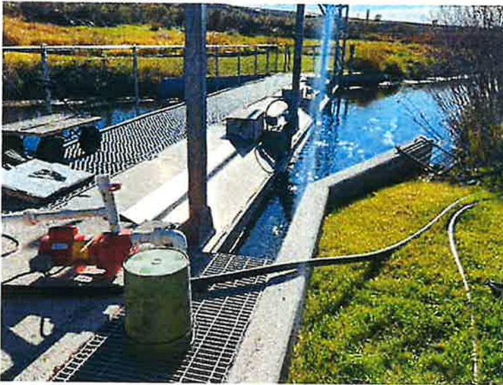
Figure 6. Pump used to pressurize a sprinkler irrigation system to irrigate 0.08 acre at the lower hatchery facility.
