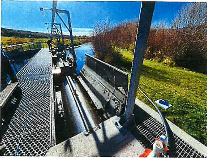
Figure 5. Fish screens and overflow structure down gradient from the broad-crested weir at the lower hatchery facility.
