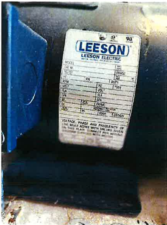
Figure 11. Pump used to pressurize a sprinkler irrigation system to irrigate 2.42 acres at the lower hatchery facility.
