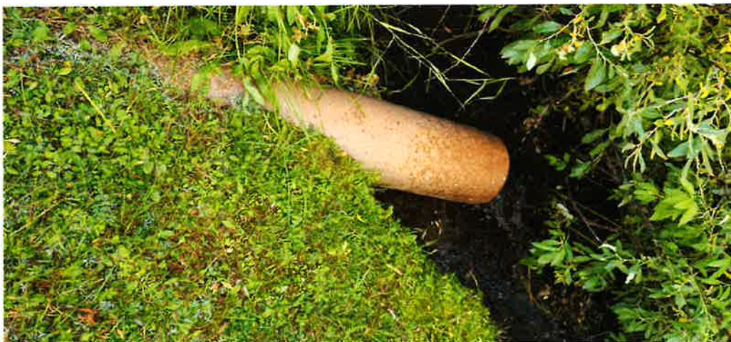
Figure 3: Bypass discharge into Williams Creek
