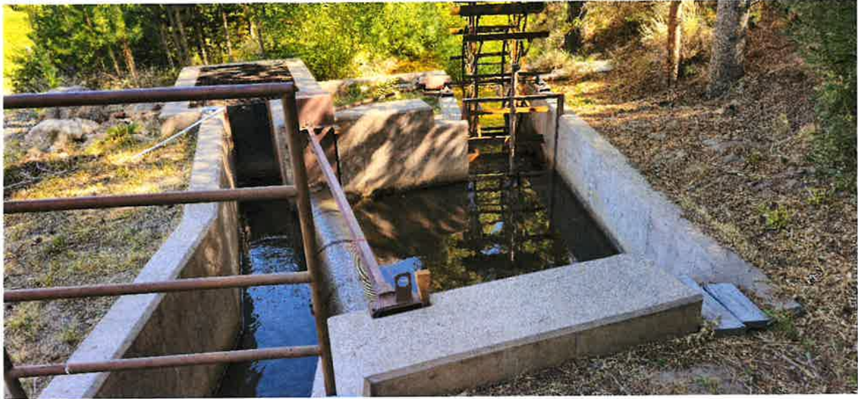
Figure 1: Fish screen with bypass (on the left side)
