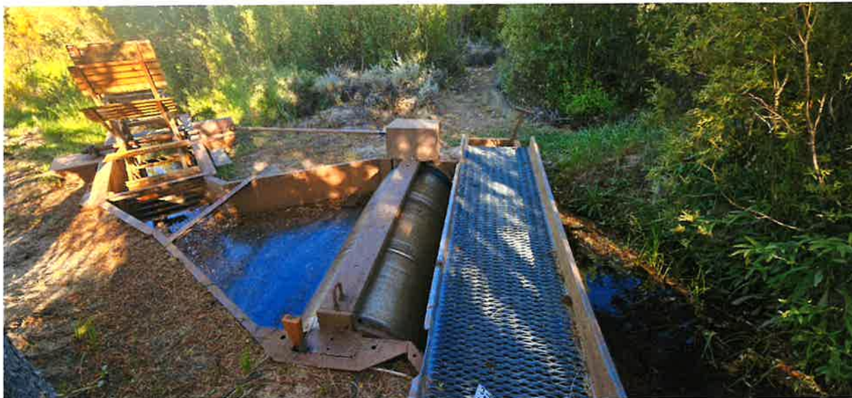
Figure 1: Fish screen with bypass (located below T-handle above walkway in photo)
