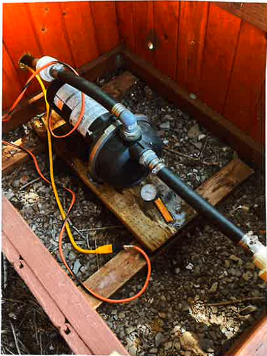
Shore-based pump to acquire water from Lake Pend Oreille
