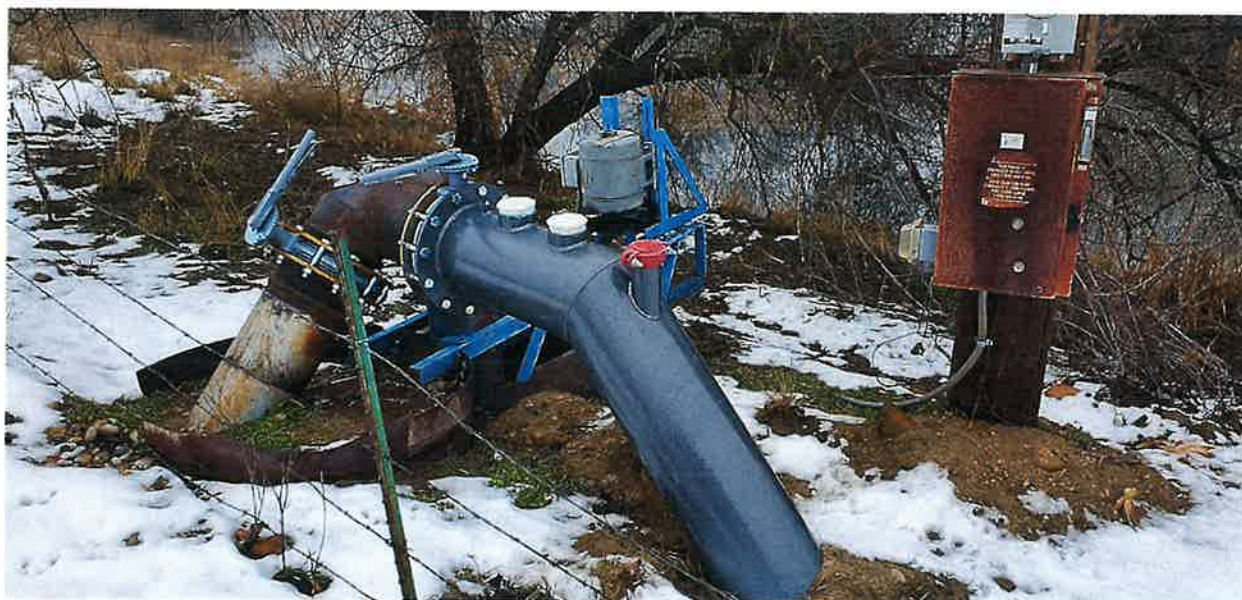
Figure 3: Pump/relift station and flooded field in background
