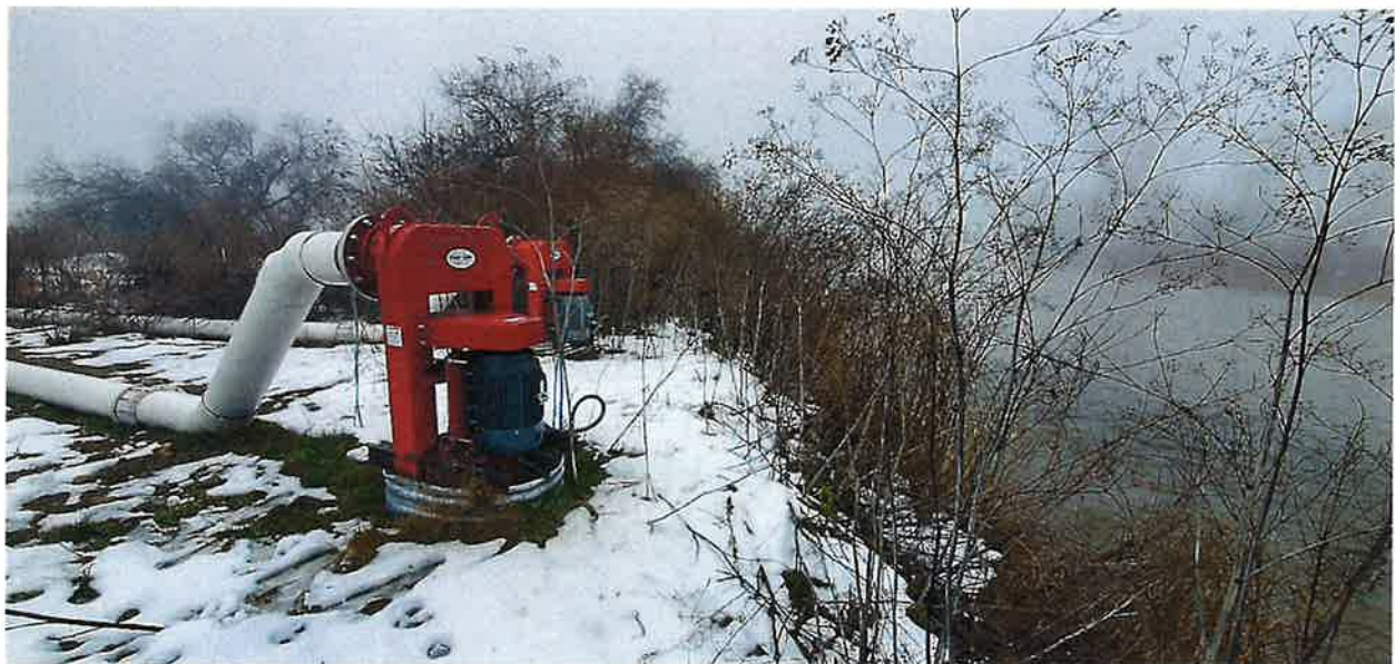
Figure 2: Pumps adjacent to river
